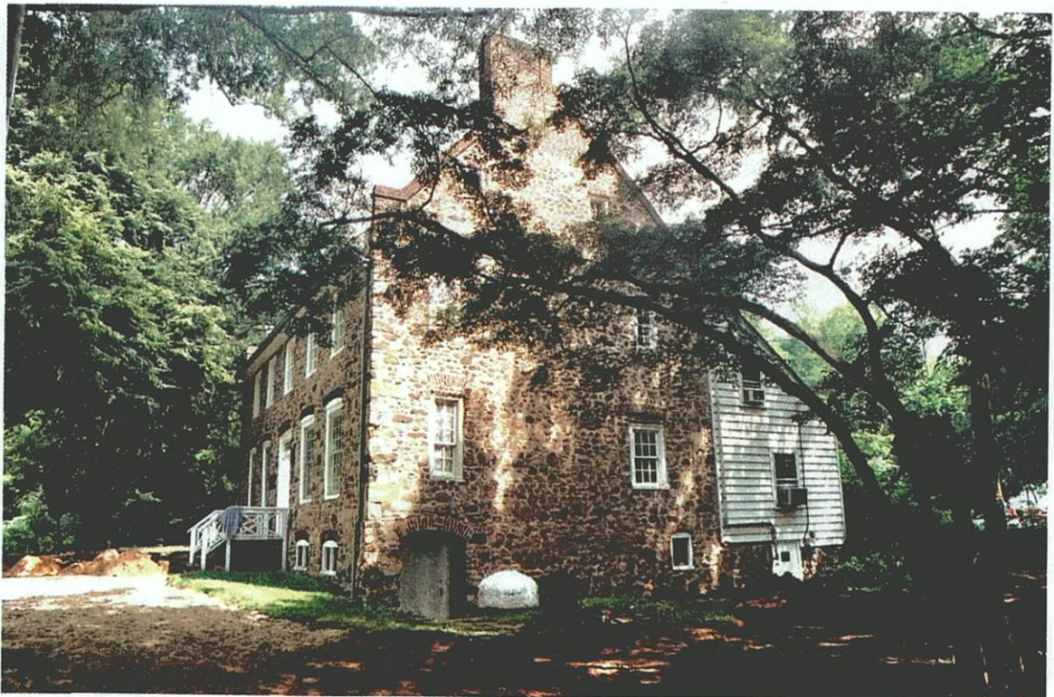
Plate C-30. South façade of the Conference House (JMA Archeological Survey Area F). Location of EU F2.7 west of door to Conference House extension at right of photograph.
