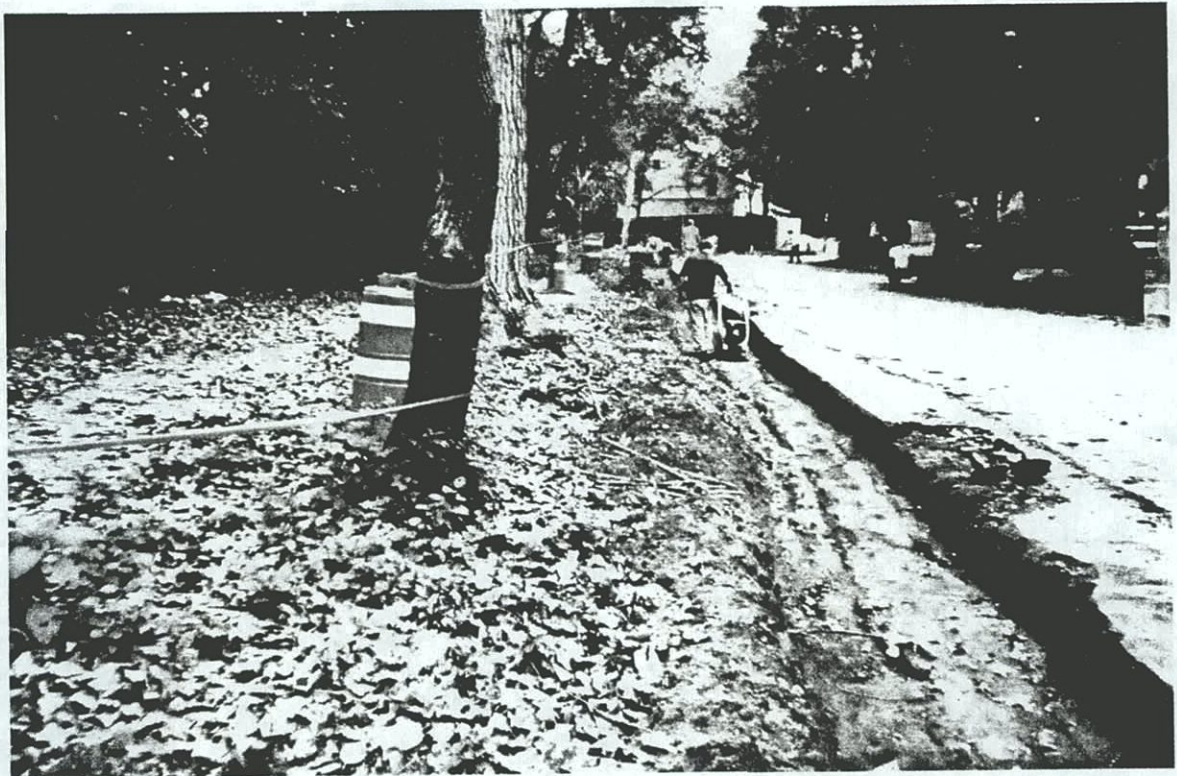
Plate C-7. Contractor compacting soil at base of Satterlee Street drainage swale trench; view north (Wood/Leven House in background).
