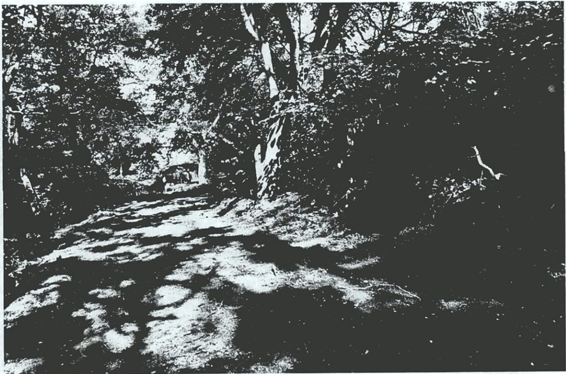
Plate C-5. Clearing and grading by the contractor at the northern end of Transect A2; view to the north.
