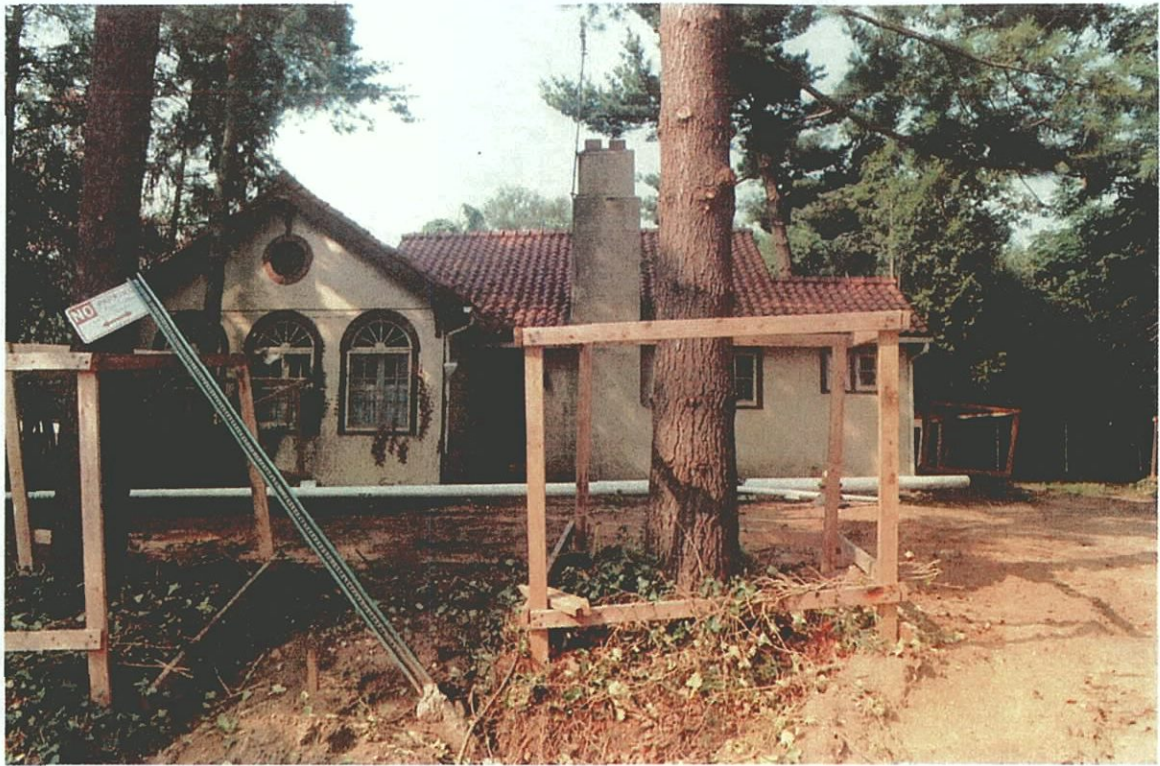
Plate C-13. Proposed Visitor's Center and yard (JMA Archeological Survey Area B3); view to the west.
