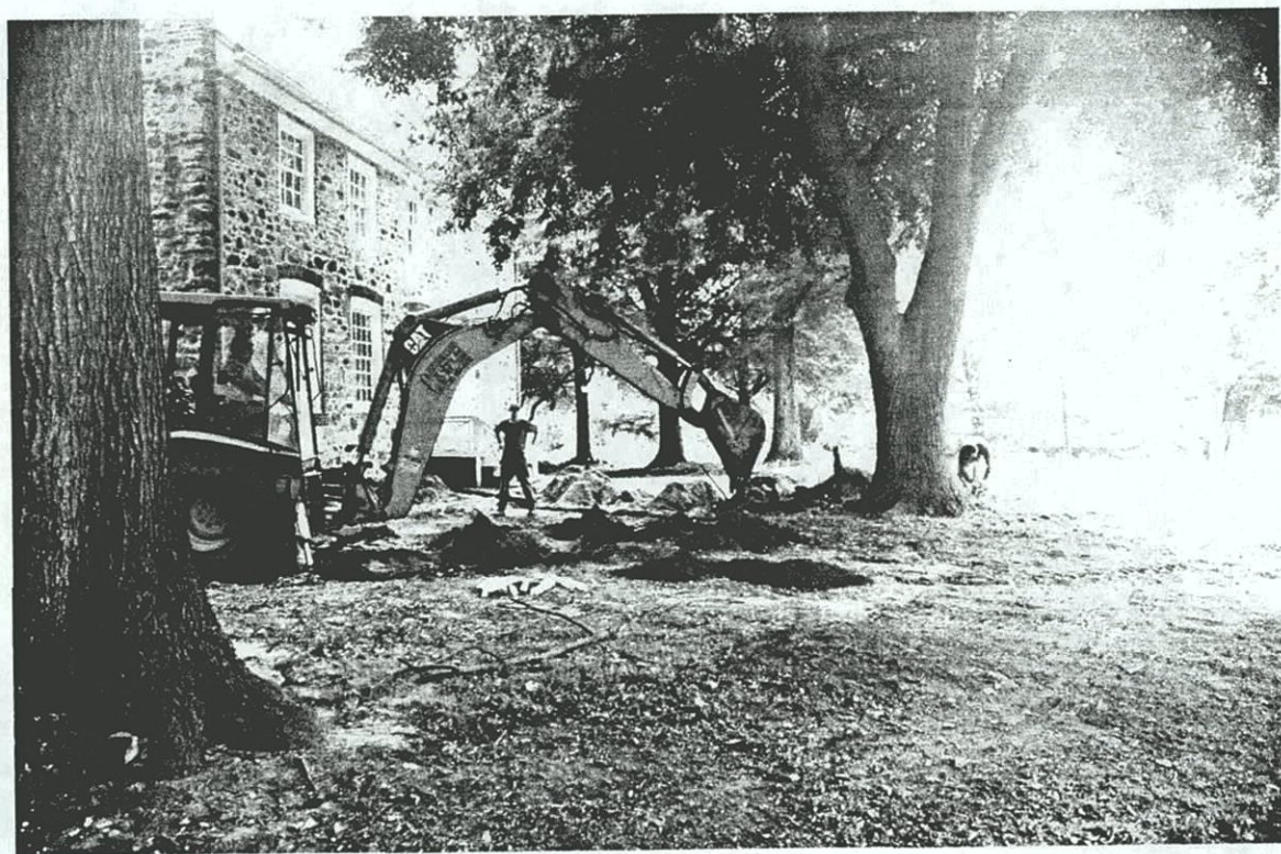
Plate C-37. JMA personnel monitoring contractor excavation of utility trench subsequent to archeological testing for STUs F4.1–F4.14; view to the northeast.
