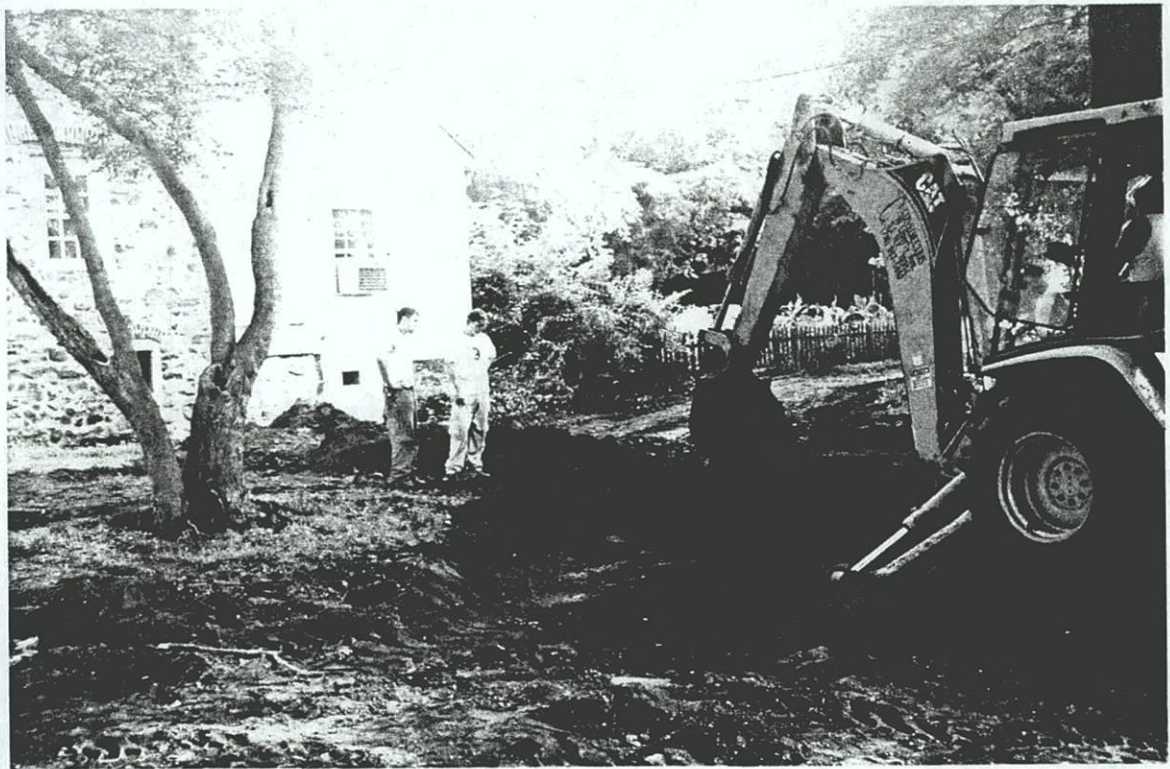
Plate C-32. JMA personnel monitoring contractor excavation of utility trench subsequent to archeological testing for STUs F2.1–F2.6; view to the northeast.
