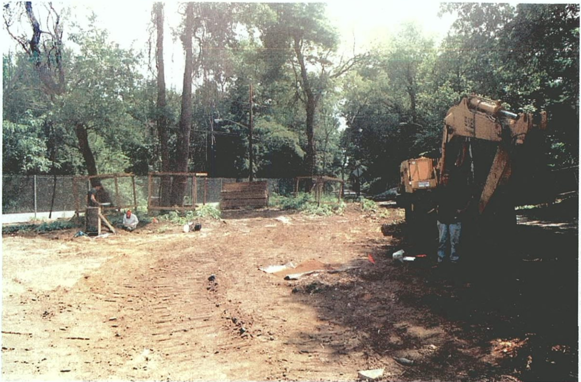
Plate C-11. Context of proposed parking lot south of Hylan Boulevard (JMA Archeological Survey Area B2) subsequent to clearing and stripping by the contractor; view to the south.
