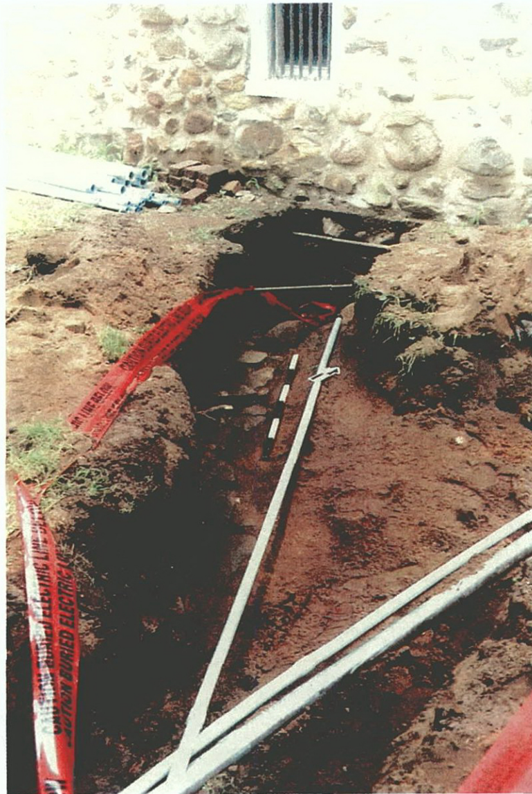
Plate C-34. Stone feature at base of utility trench documented during monitoring and subsequent to excavation of STUs F2.1–F2.6; view to the north.
