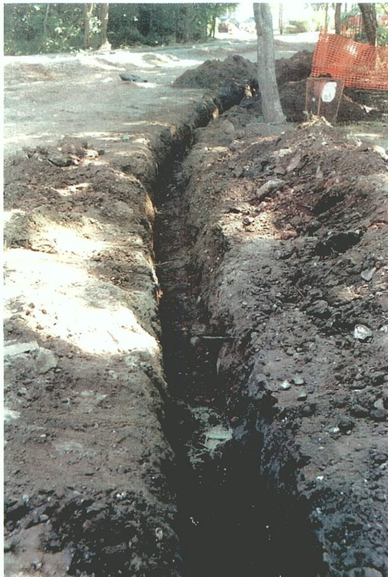
Plate C-41. Utility trench east of the Conference House subsequent to excavation of STUs F5.2–F5.22; view to the east.
