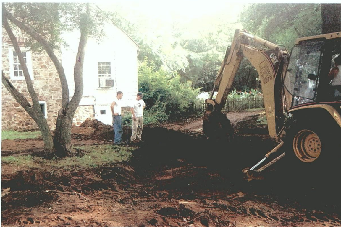
Plate C-32. JMA personnel monitoring contractor excavation of utility trench subsequent to archeological testing for STUs F2.1–F2.6; view to the northeast.
