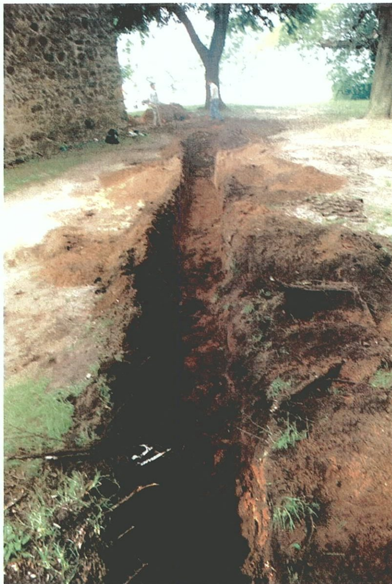
Plate C-38. Utility trench north of the Conference House subsequent to excavation of STUs F4.1–F4.14; view to the west-southwest.
