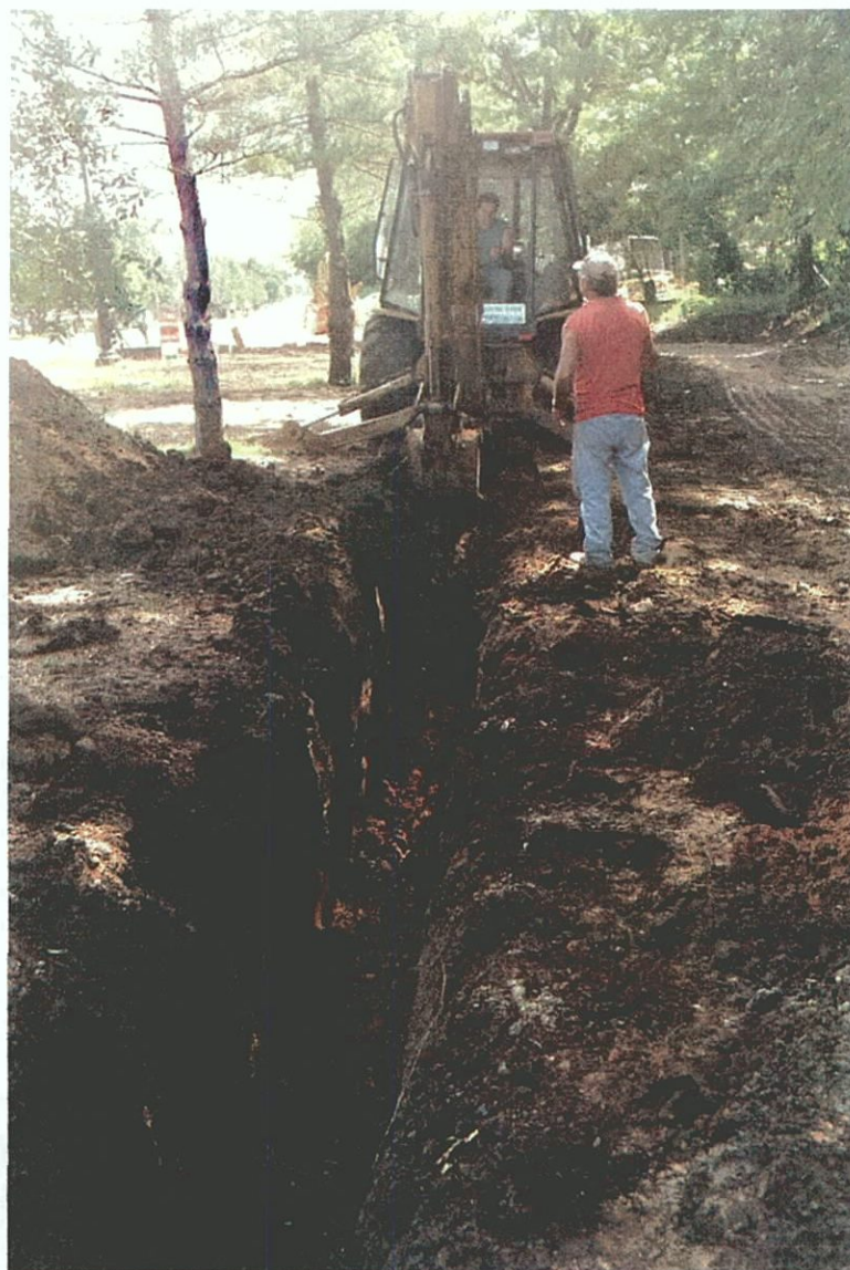
Plate C-9. Excavation of trench by the contractor for water line (JMA Archeological Survey Area B1); view to the east.
