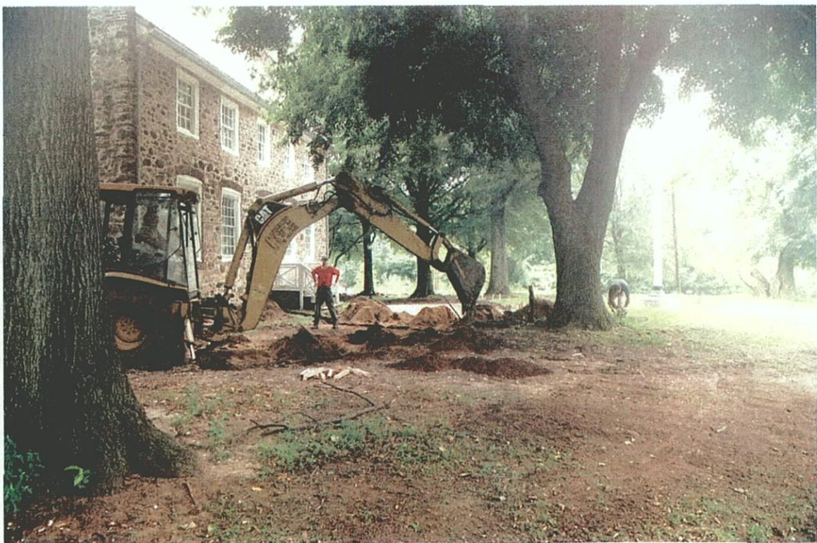
Plate C-37. JMA personnel monitoring contractor excavation of utility trench subsequent to archeological testing for STUs F4.1–F4.14; view to the northeast.
