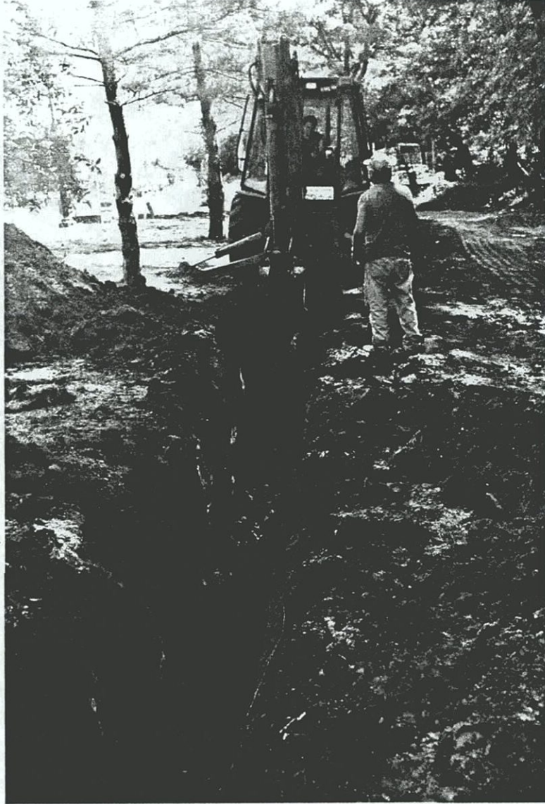
Plate C-9. Excavation of trench by the contractor for water line (JMA Archeological Survey Area B1); view to the east.
