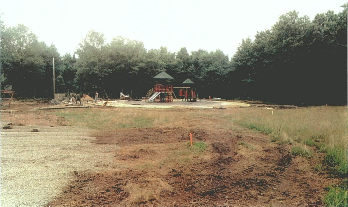
Plate C-24. Playground during construction within JMA Archeological Survey Area D1; view to the south.
