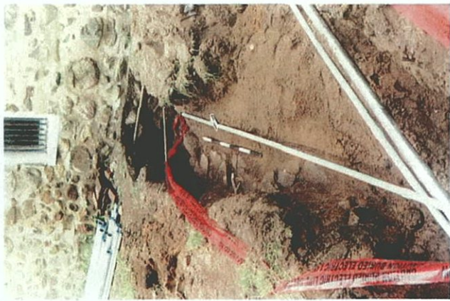
Stone feature observed in utility trench extending south from Excavation Unit F2.7.
