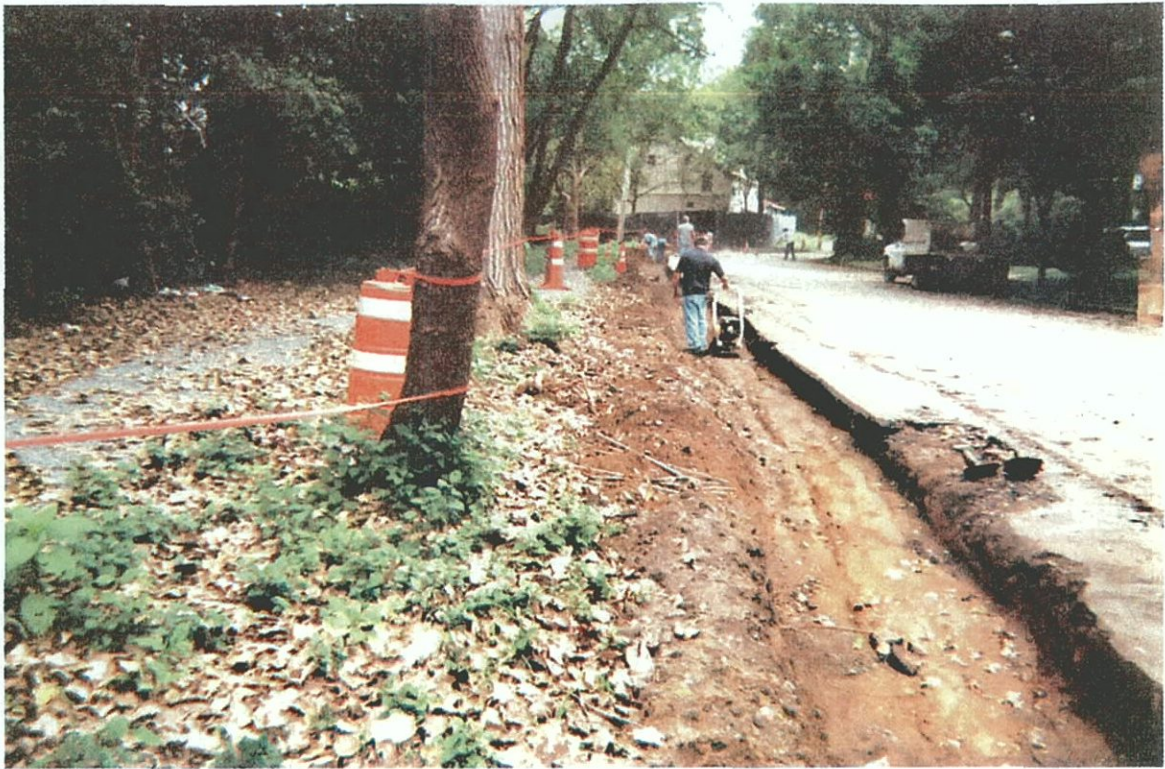
Plate C-7. Contractor compacting soil at base of Satterlee Street drainage swale trench; view north (Wood/Leven House in background).
