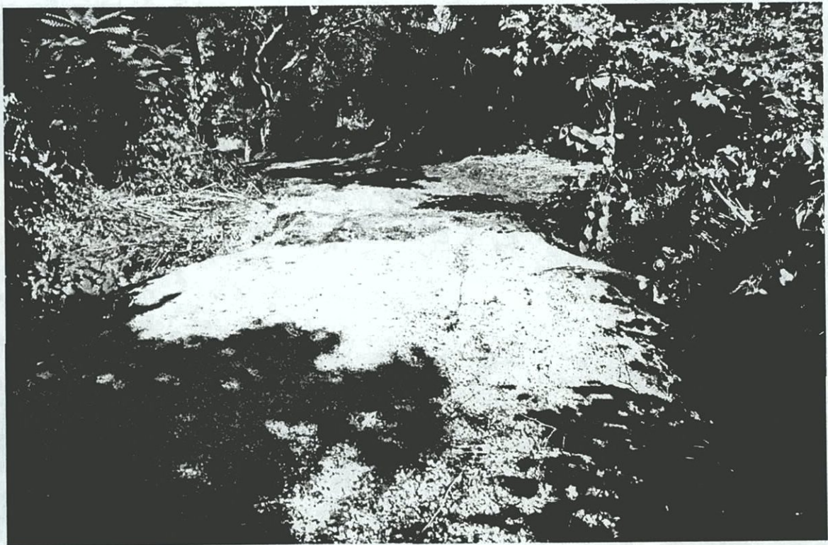
Plate C-4. Drainage culvert and gravel installed by the contractor at swale-crossing within the northern portion of Transect A2; view to the northwest.
