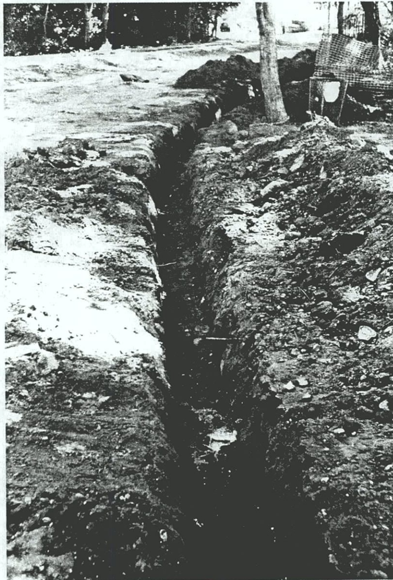
Plate C-41. Utility trench east of the Conference House subsequent to excavation of STUs F5.2–F5.22; view to the east.
