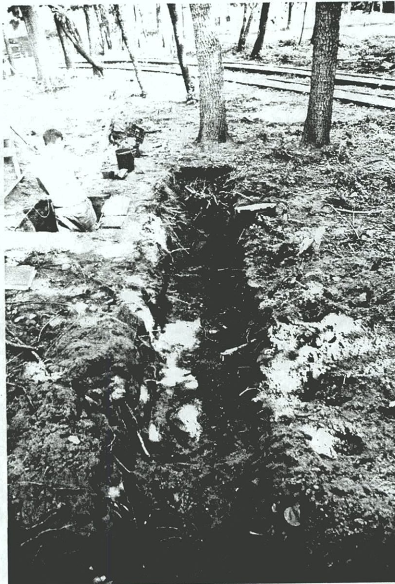
Plate C-39. JMA personnel excavating EU F5.1 (left) adjacent to utility trench excavated by contractor in east yard of the Conference House; view to the south.
