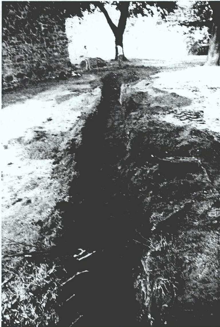
Plate C-38. Utility trench north of the Conference House subsequent to excavation of STUs F4.1–F4.14; view to the west-southwest.
