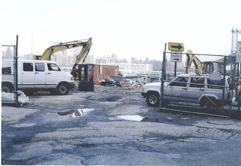
Photograph 12: Block 16, looking north from Plymouth Street showing area under construction at western end of block.
