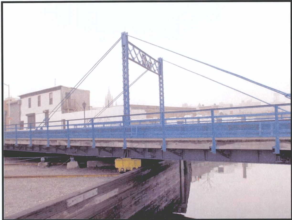
Plate 3.11. Gowanus Canal Assessment of Eligibility: View north of the Carroll Street Bridge (Photographer: James Lee, November, 2003)[ HRI Neg. # 03070 D1-46].
