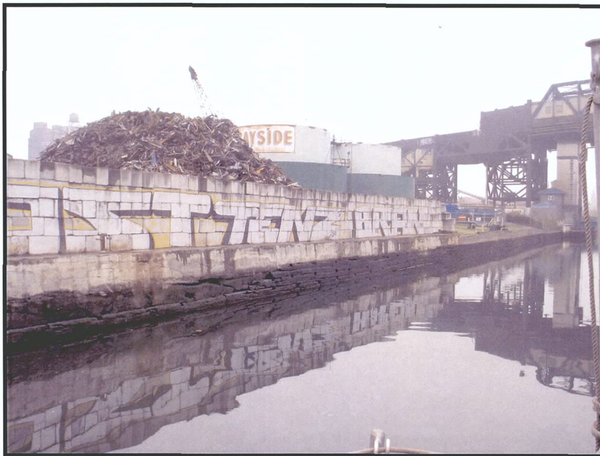
Plate 3.14. Gowanus Canal Assessment of Eligibility: View northeast near the 11th Street basin showing concrete additions to the cribwork bulkhead face (left) and new timber face on cribwork bulkhead (right). The New York Transit Authority trestle is visible in the background (Photographer: Thomas Flagg , November 2003) [Source: Raber Associates].
