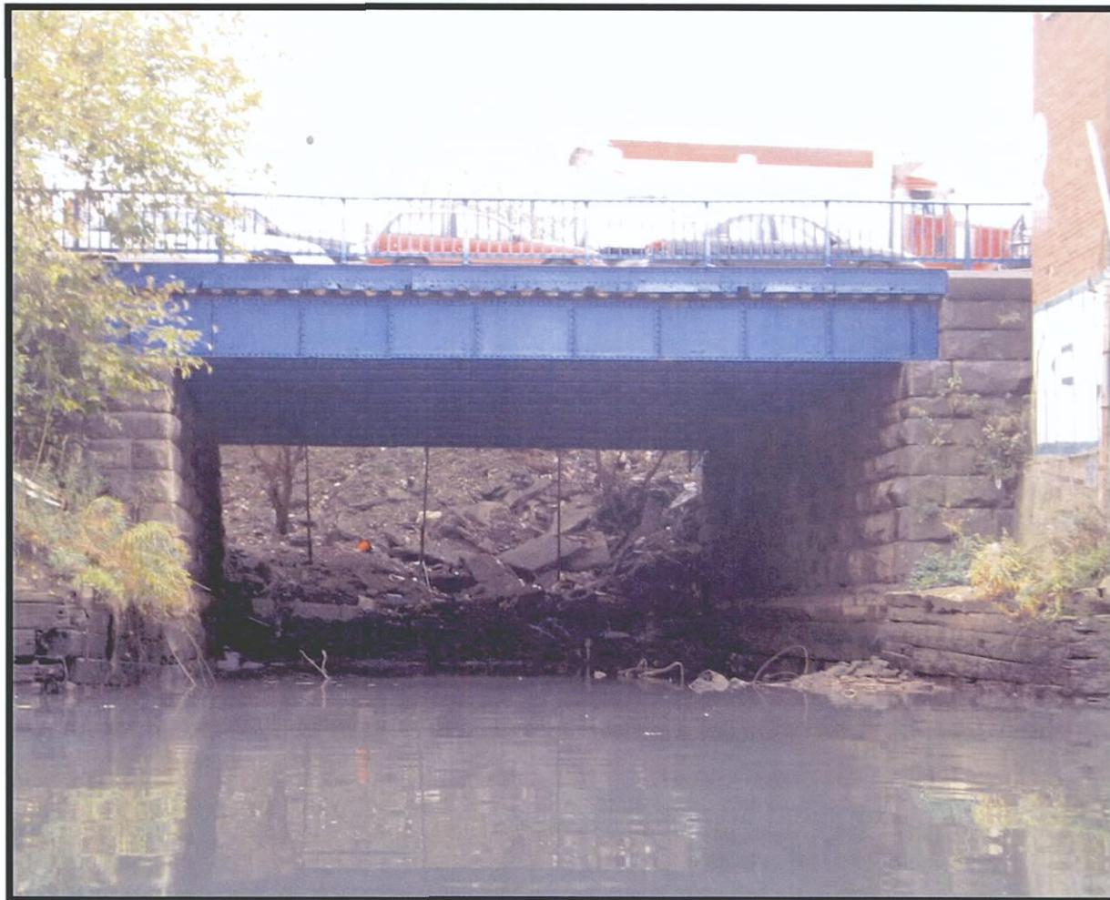
Plate 2.8. Gowanus Canal Assessment of Eligibility: View southeast of Third Avenue Bridge. The filled 5th Street basin is visible in the background (Photographer: Thomas Flagg, November 2003) [Source: Raber Associates].
