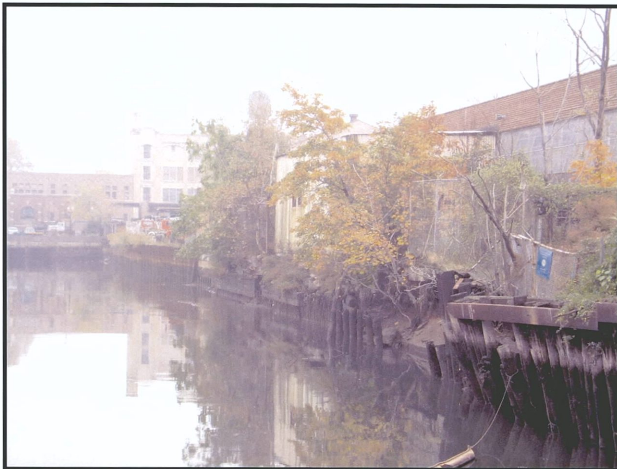
Plate 3.10. Gowanus Canal Assessment of Eligibility: View northeast towards the end of the canal, with timber sheetpile (right) and steel sheetpile (left center) bulkheads, and concrete bulkhead at the end of the canal (left) (Photographer: Thomas Flagg, November 2003) [Source: Raber Associates].
