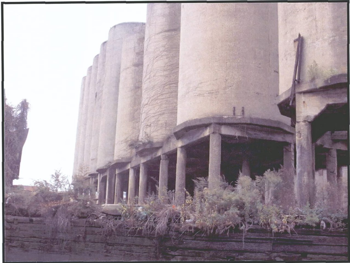
Plate 3.21. Gowanus Canal Assessment of Eligibility: View southwest of Burns Bros. Coal Pockets and timber cribwork bulkhead near the head of the 4th Street Basin (Photographer: Thomas Flagg, November 2003) [Source: Raber Associates].
