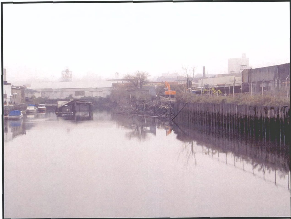
Plate 3.5. Gowanus Canal Assessment of Eligibility: View southeast of the 6th Street basin. A steel sheetpile bulkhead is seen at the right of the view, with a collapsing timber bulkhead visible beyond (center right of view). An intact timber bulkhead (center left of view) and a steel bulkhead (left) can also be seen (Photographer: Thomas Flagg , November 2003) [Source: Raber Associates].
