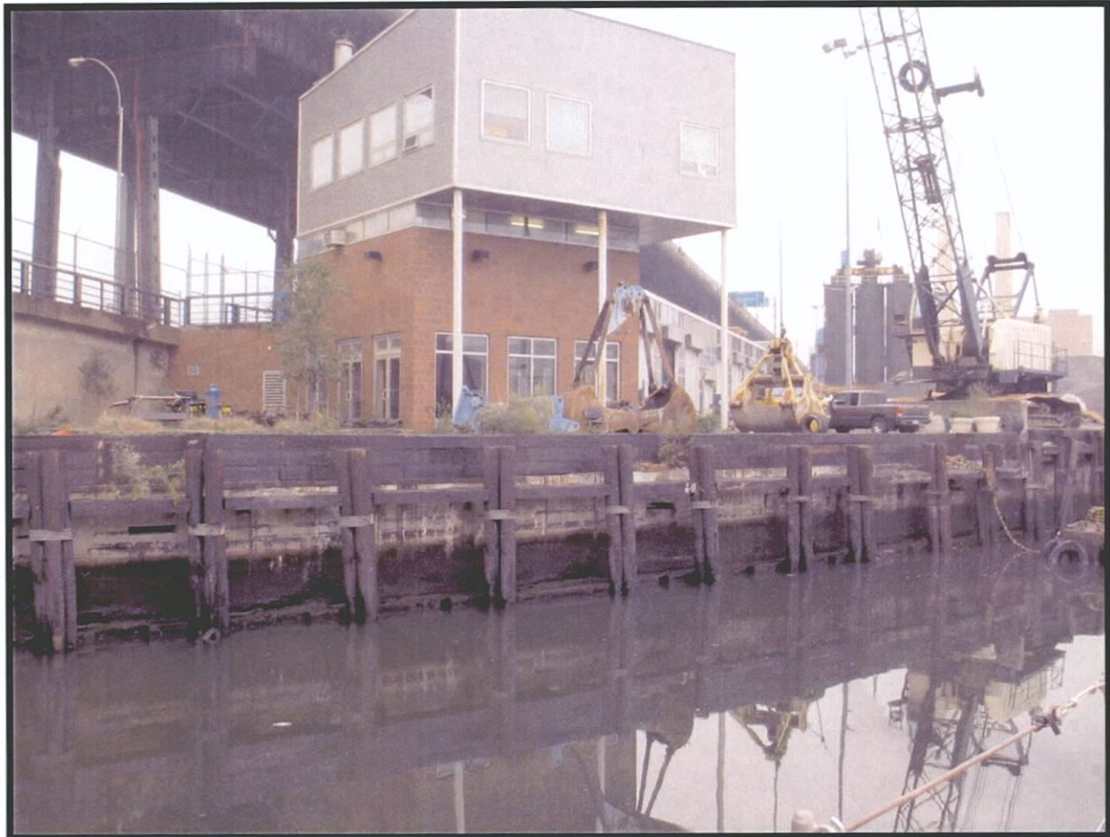
Plate 3.1. Gowanus Canal Assessment of Eligibility: View south of recent bulkhead at 14th Street, with concrete face above possible cribwork cut off at the mean low water mark (Photographer: Thomas Flagg, November 2003).
