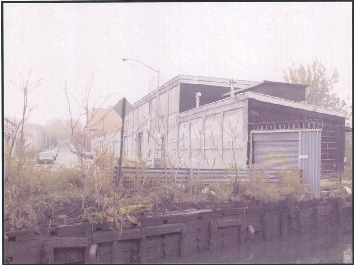
Plate 3.9. Gowanus Canal Assessment of Eligibility: View northwest of the intact timber crib-work bulkhead at the end of 1st Street, with a 1916 concrete oil terminal structure (Photographer: Thomas Flagg, November 2003) [Source: Raber Associates].
