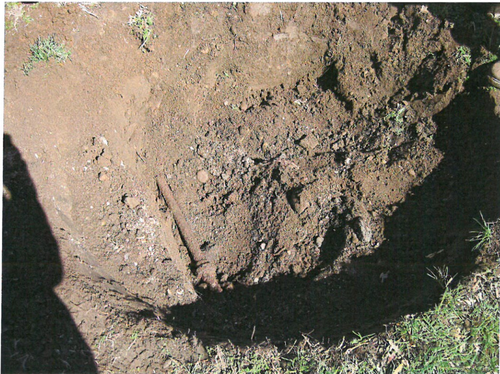
Figure 11: T03A: gas pipe encountered
