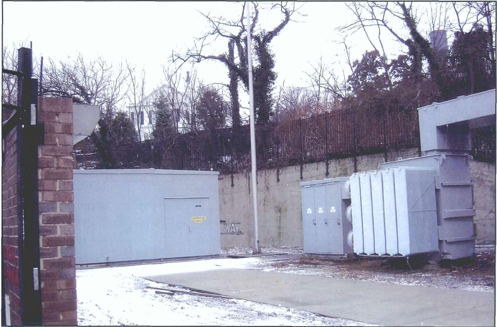
Photo 4. Interior view of substation, facing southeast. Note the existing concrete walkways and foundations. Note the existing concrete walkways and foundations. The switches and generating equipment visible in the photograph are connected via underground ductbanks and conduits running beneath the concrete paths.
