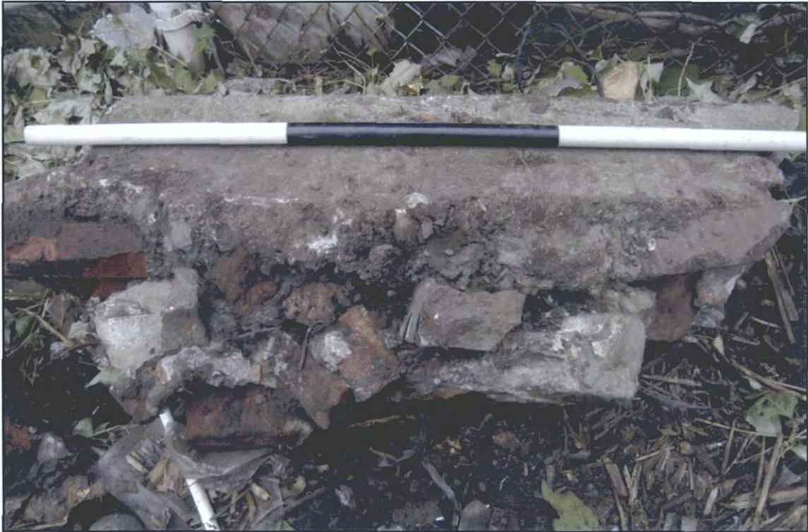
Photo 4: Section of Concrete Curb Showing Fragmentary Bricks and Mortar Base.
