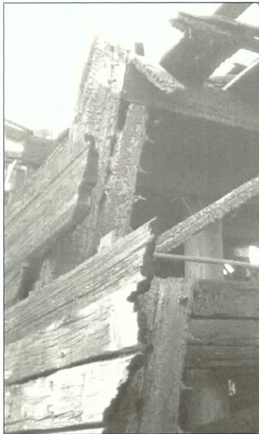
Figure 5-99. Inner wing frame. Note upper deck at top of photo, also seen in Figure 5-96. Starboard wing view to the north (forward).
