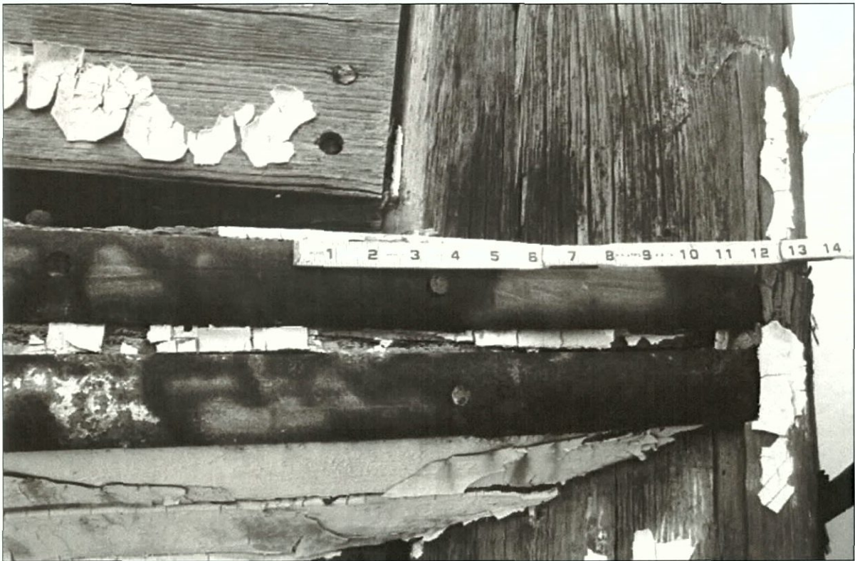
Figure 7-57. Main rub rail where it meets the starboard side of the stem. Note iron half-round caps.
