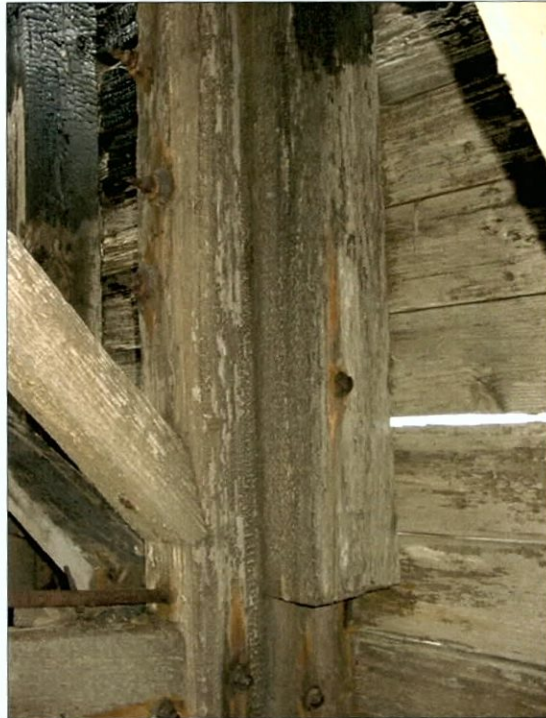
Figure 5-114. Mortise and tenon joint, outer wall, port wing. View to the southwest (aft).
