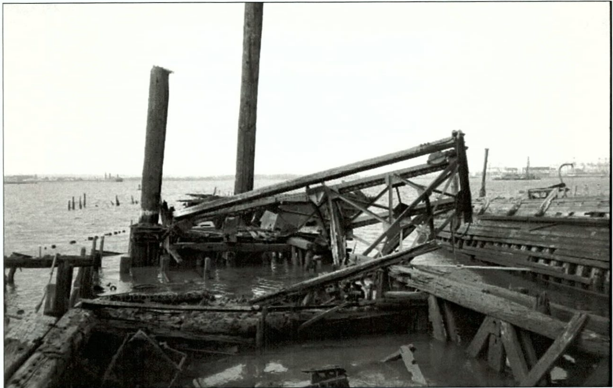
Figure 4-62. Aft end of V36, showing collapsed A-frame and spud poles. View to the north.
