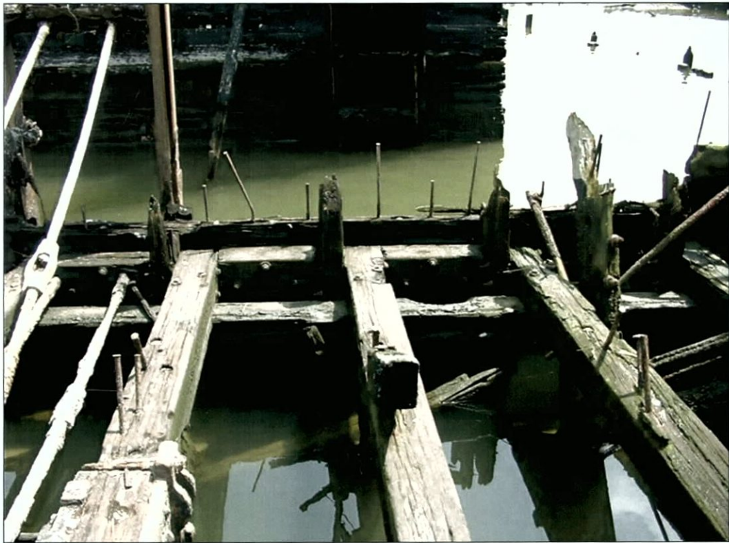
Figure 5-54. Vessel side framing on northern exposed end of V1. Note spacing and chocks. View to the east.
