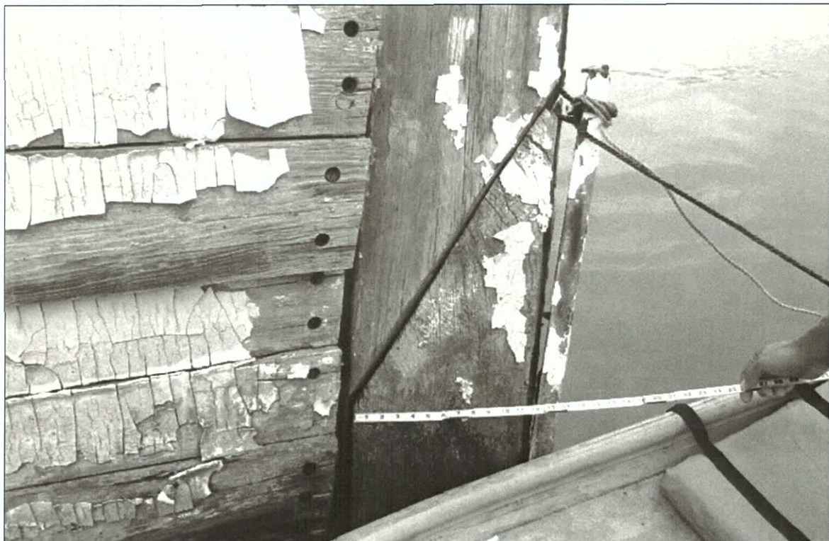
Figure 7-44. Close-up of stern showing scarp joint. Also note stern band. View to the east (port).
