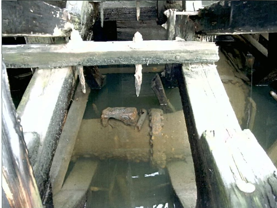
Figure 5-156. Outlet pipe. Outlet in upper right of image corresponds with the outer hull fitting in Figure 5-148. Port wing, view to the west (port).
