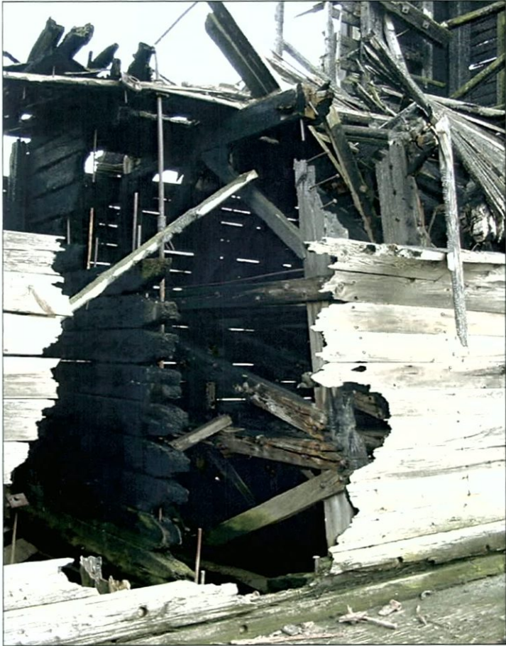
Figure 5-103. General view of wing truss. Starboard, view toward aft quarter of V1 (southeast).
