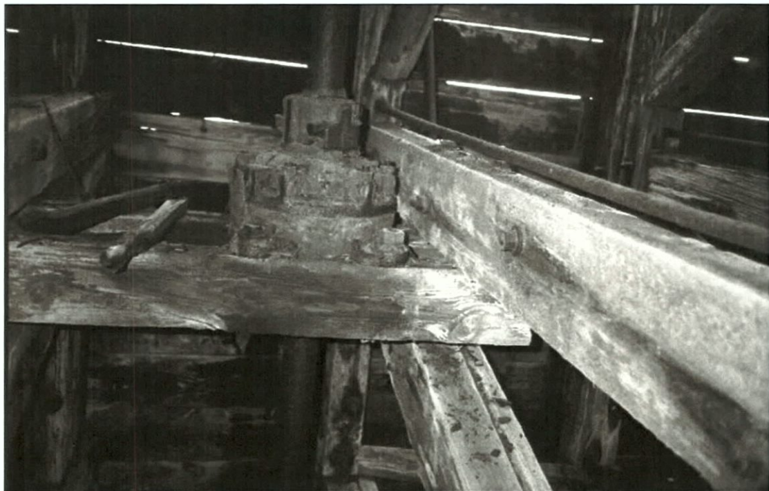
Figure 5-161. A pair of longitudinal stringers spanning two frames provides support for the vertical actuator shafts for the gate valves, floodgates, and pump.
