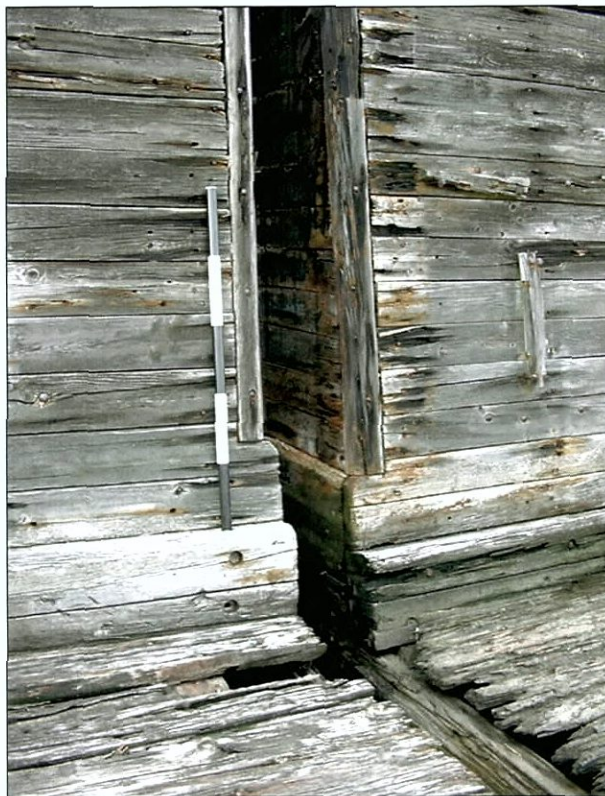
Figure 5-129. Port wing, aft inner corner, showing half round corner post. View to the west (port).
