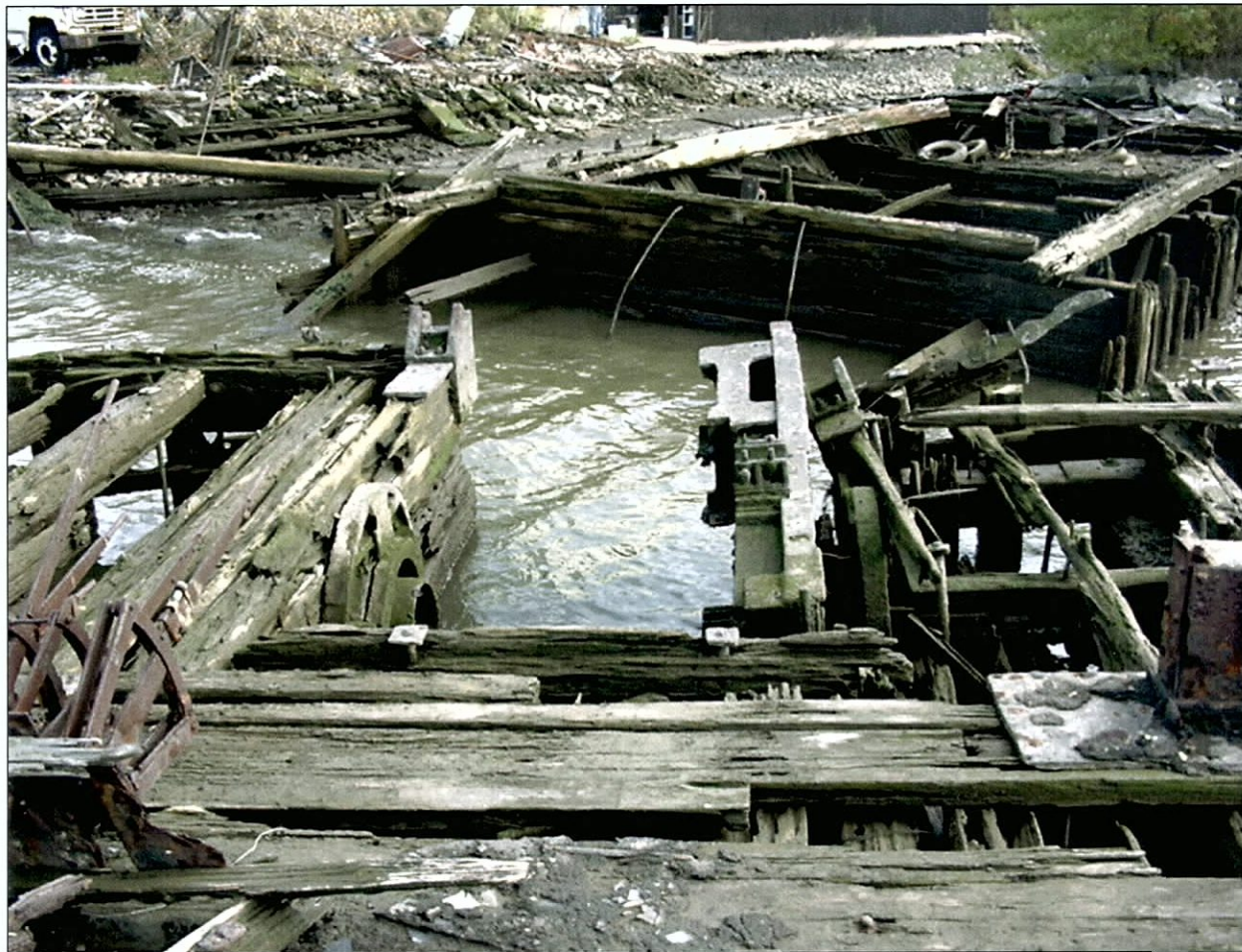
Figure 4-28. Ladder well in the bow of V36. Note remains of A-frame attachment. View to the south (forward).
