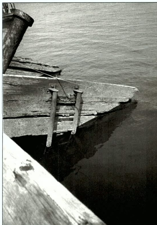
Figure 7-91. Cargo hold access ladder on aft end of hatch coaming. View to the north.
