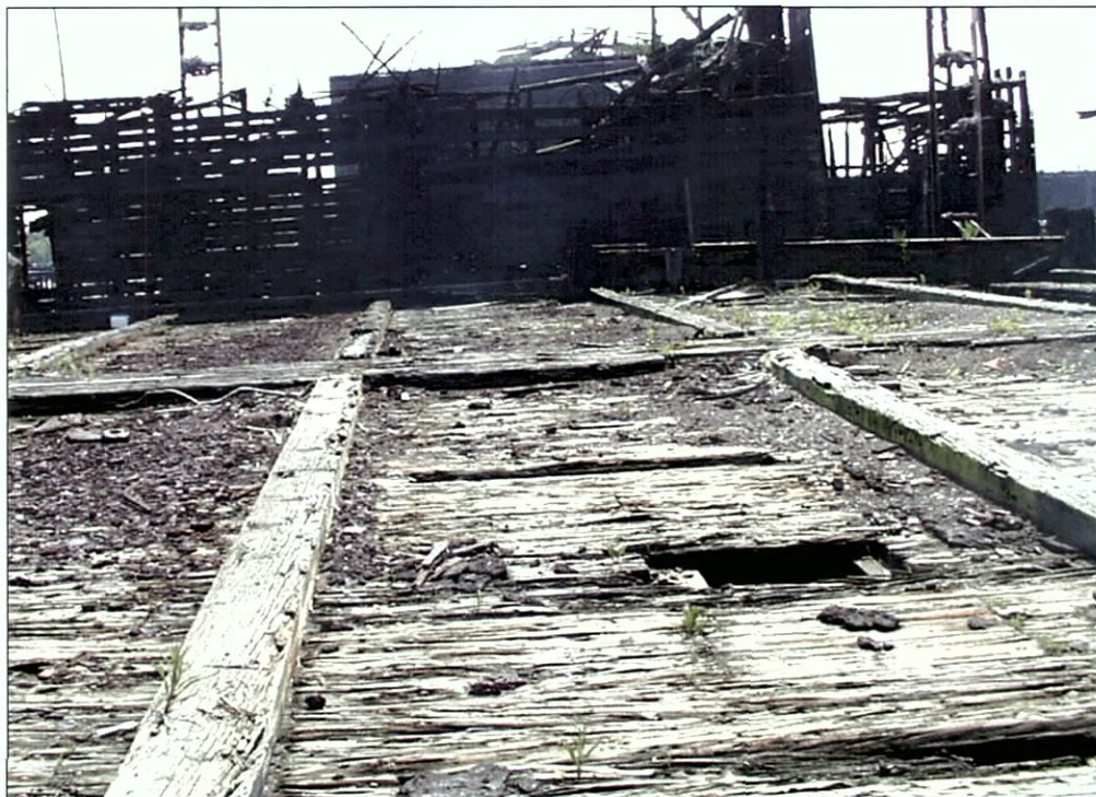
Figure 5-178. Main deck looking aft (south). Note large amount of debris.
