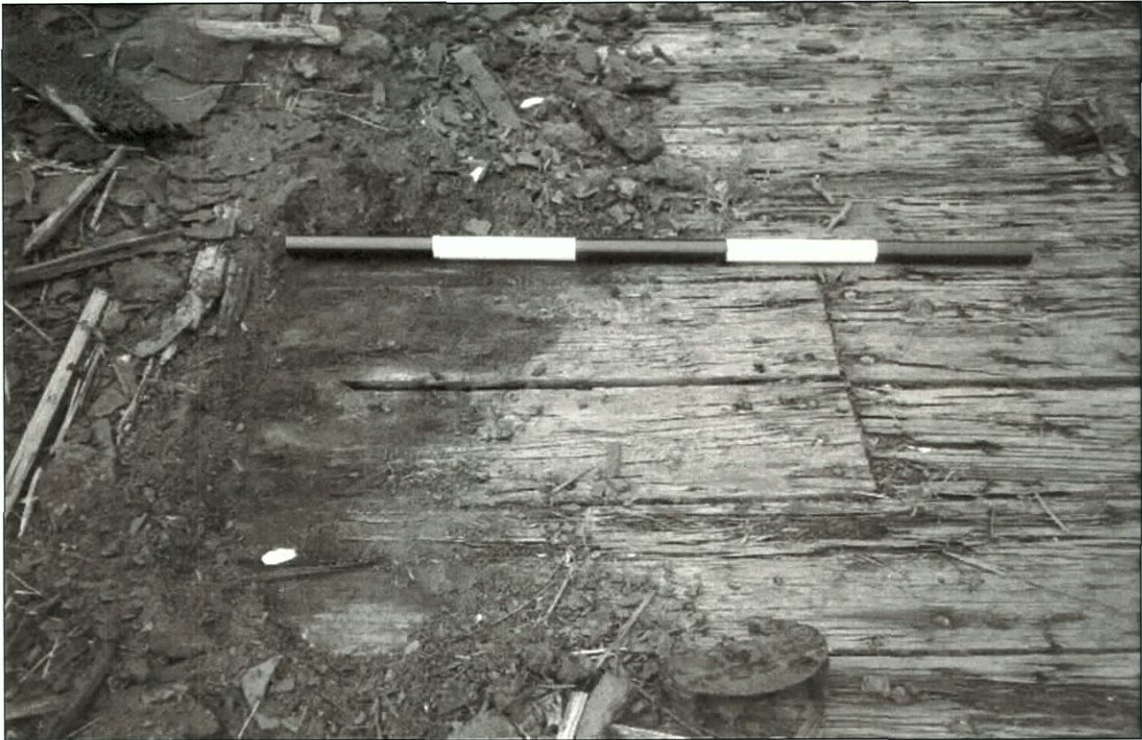
Figure 5-171. Small section of replaced deck plank on main deck. Note different fasteners on patch.
