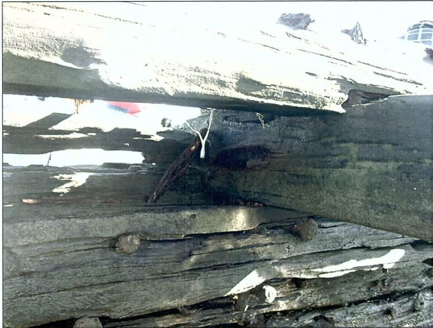
Figure 6-95. Port side view looking port (east) showing deck beam, waterway, and clamp.
