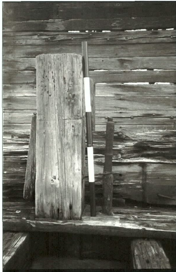
Figure 5-71. Cinch bolt on forward port bitt. Cradle has eroded or been removed. Lag bolt extends to framing below. View to the west.
