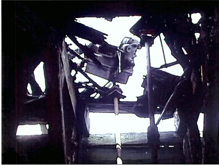
Figure 5-152. Gate valve actuator motor. Note shaft.
