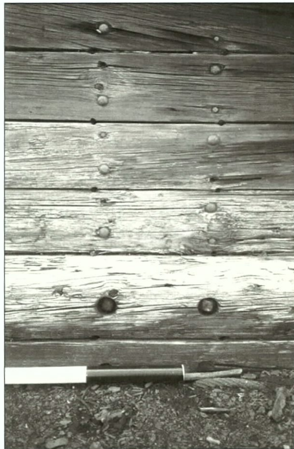
Figure 5-124. Wing chine and wing plank fastener pattern at bulkhead location. Note two types of fasteners. View to the west (port).
