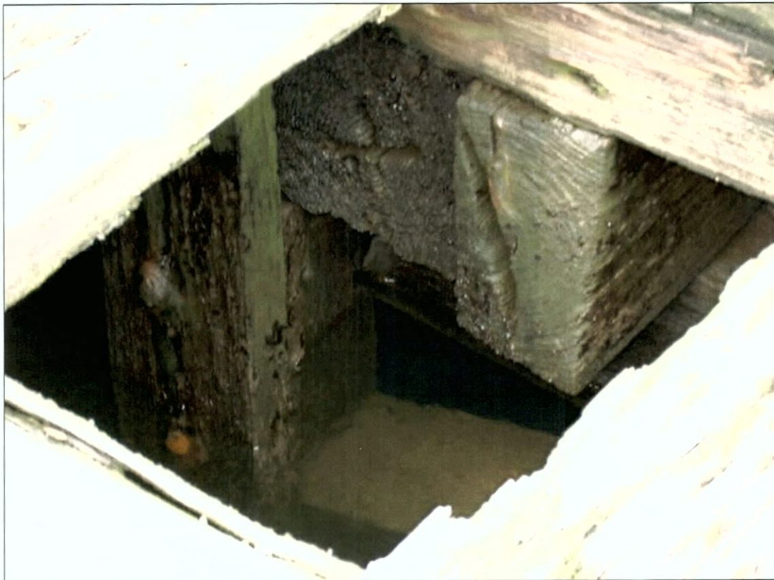
Figure 5-75. View of bitt structure at deck beam 6. View toward northwest (forward port). Note stringer to right of vertical stanchion, chock to right of stringer, and transverse support below stringer and chock.
