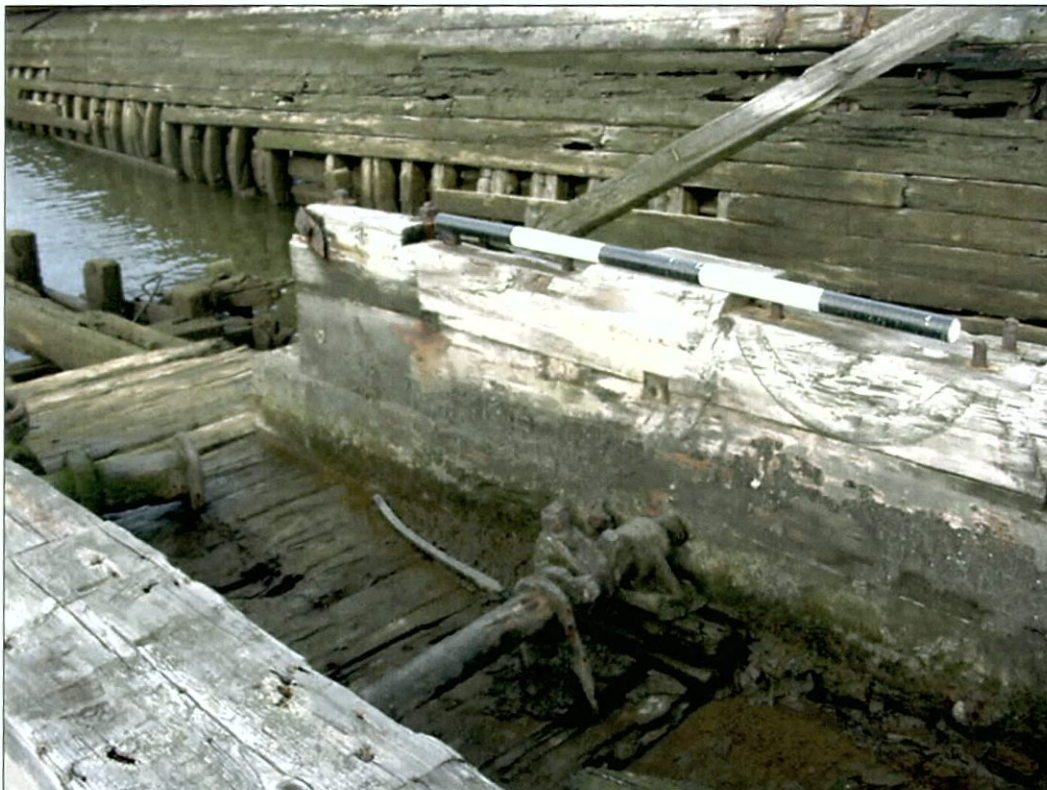
Figure 4-53. Close-up of port side cable mount. View to the northeast (port aft).
