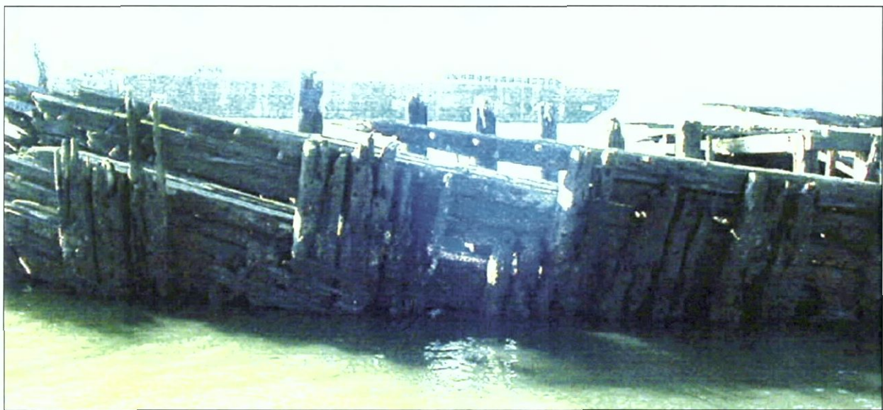
Figure 6-106. Port side, forward, framing (colors exaggerated to enhance definition). View to the southwest.
