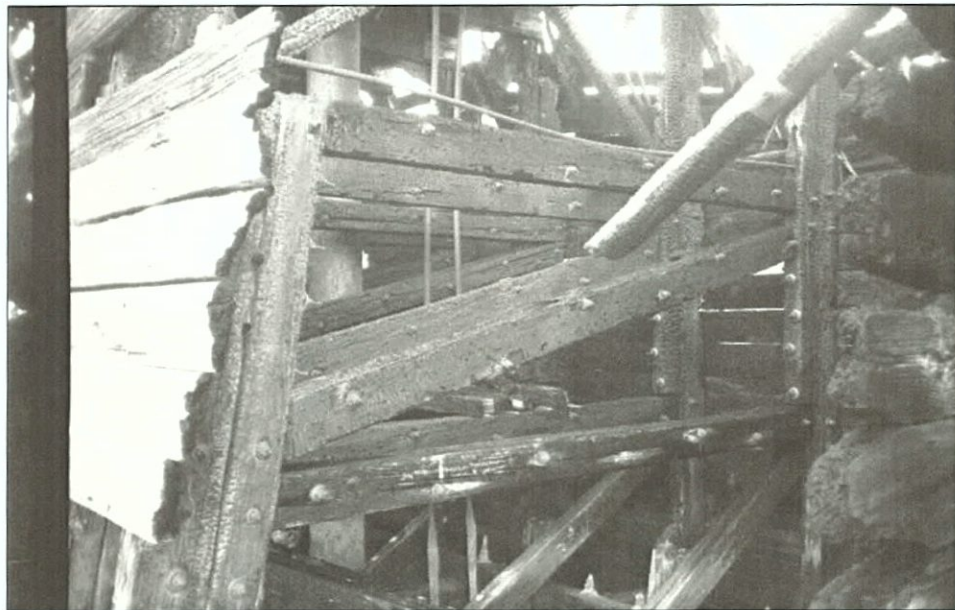
Figure 101. Wing truss above main deck level. Starboard wing. View to the northeast.
