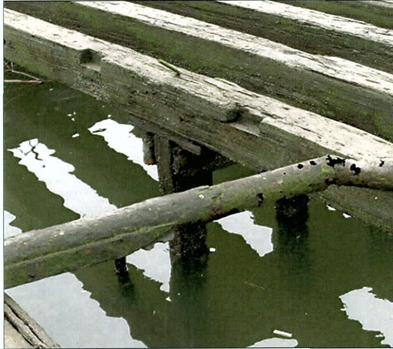
Figure 6-98. Stanchion detail on aft edge of forward cargo hatch. Note presence of stringers, cut just forward of the stanchion, the caps, and the absence of an iron reinforcing strap.
