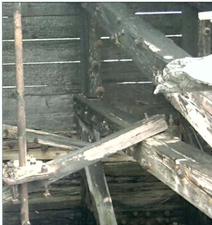
Figure 5-109. Starboard wing outer wall, view to the east. Note joint against outer hull, at center of photo.
