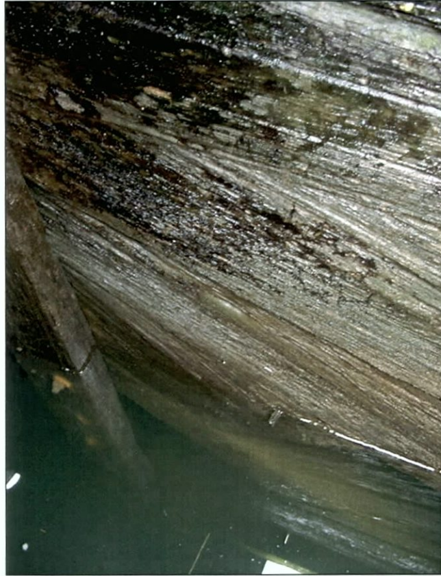
Figure 5-59. Confluence of trusses at centerline bulkhead (T1). View from port toward centerline, to the southeast.
