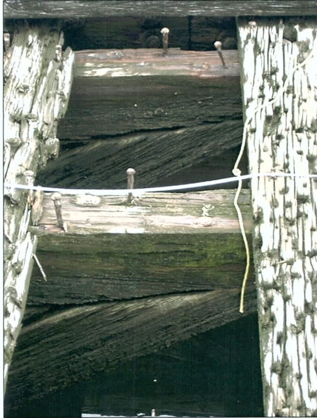
Figure 5-61. Truss 6 at main deck. Note end of triangular chock at left. View to the north (forward).
