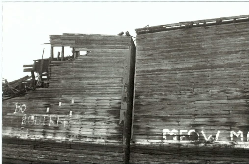
Figure 5-126. Outer wall, port wing. Note planking dimensions. View to the east (starboard).
