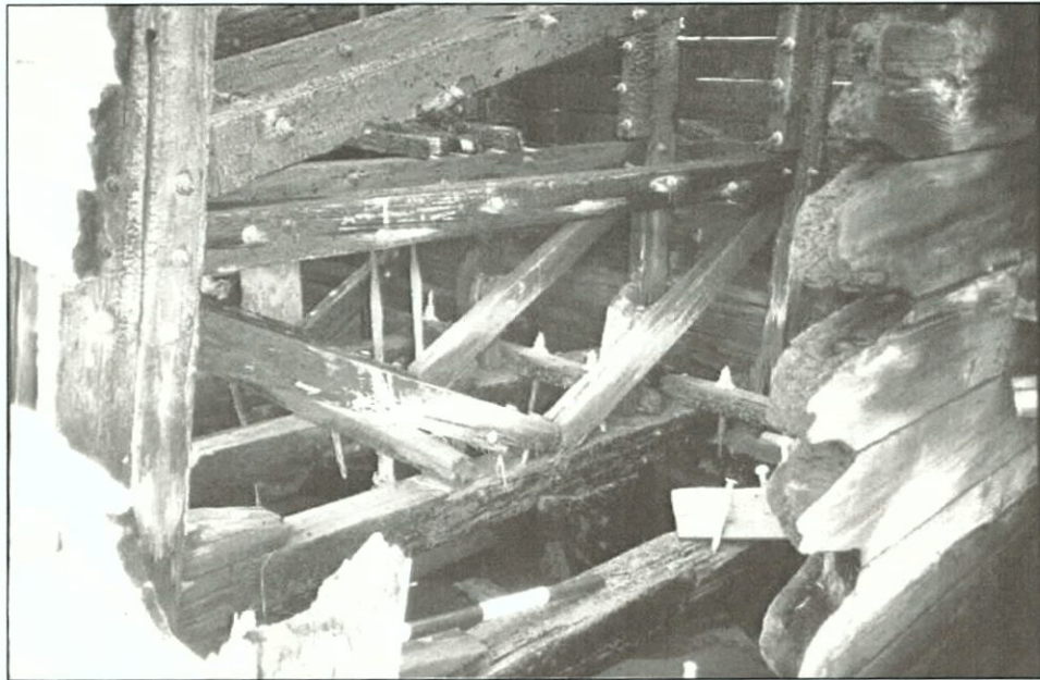
Figure 5-100. Wing truss at main deck level. Starboard wing. View to the northeast.
