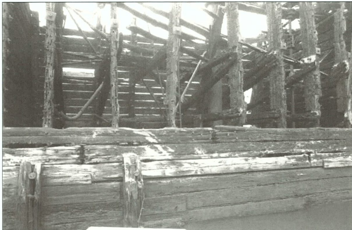
Figure 5-32. Close-up of starboard side, view to the southwest. Note outer hull planking with butt joints.
