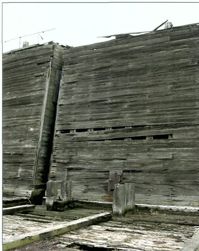
Figure 5-120. Port wing aft. Note chine logs at base and differing size planking, especially larger scantling planks at top. View to the southwest (port).
