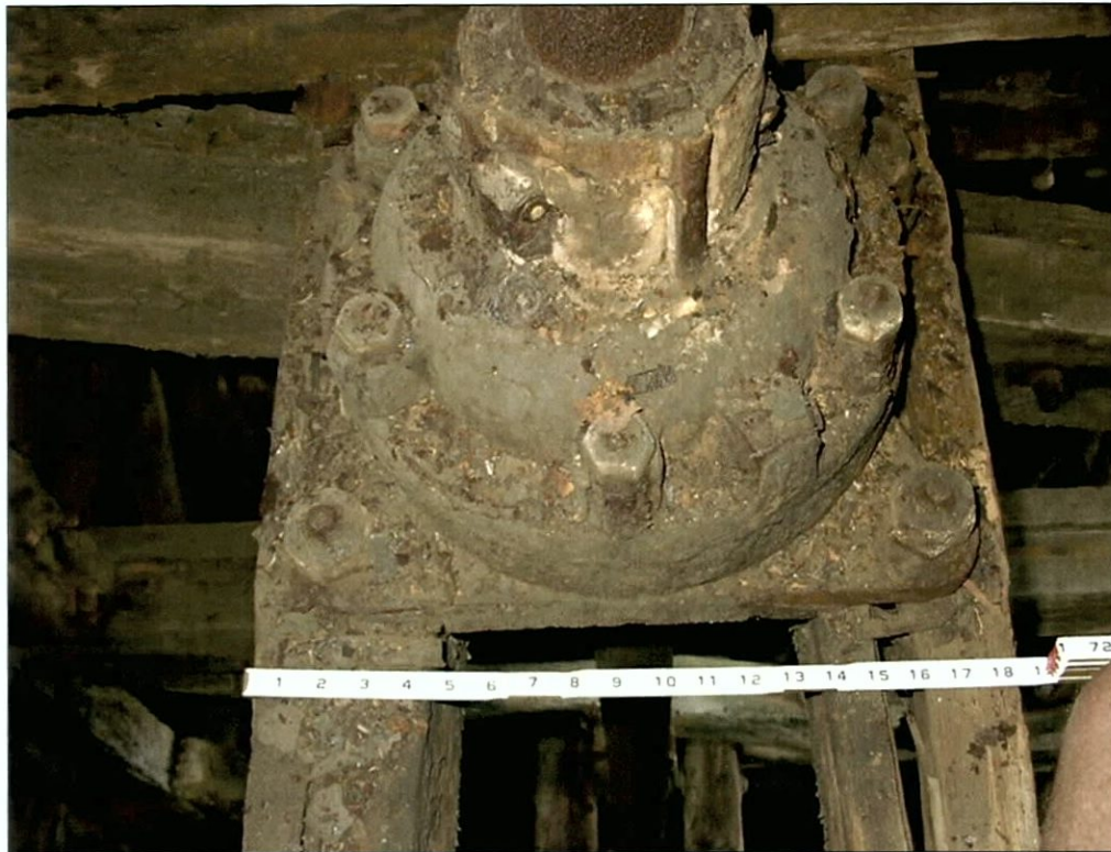
Figure 5-162. Close-up of support structure for pump drive shaft.
