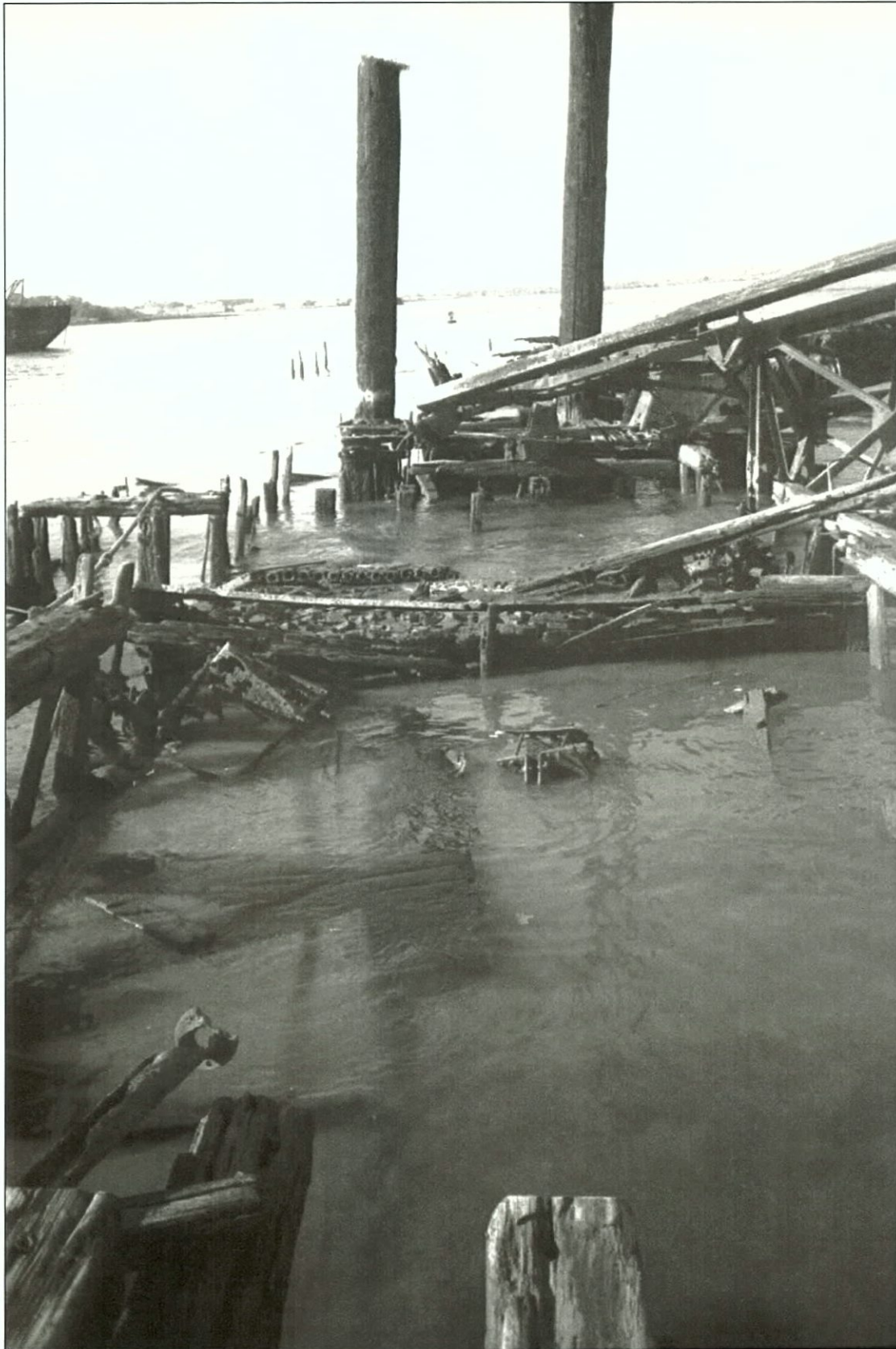
Figure 4-25. V36, general view of the main deck. View to the north (aft). Note spuds and collapsed A-frame.
