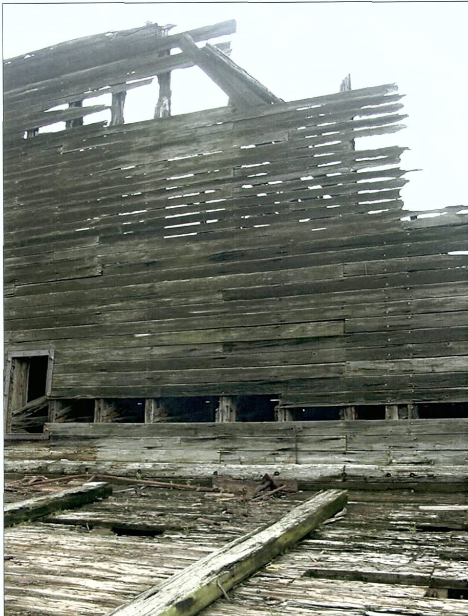
Figure 5-118. Port wing showing inner wing wall planking. Note change in dimension toward top. View to the west (port).
