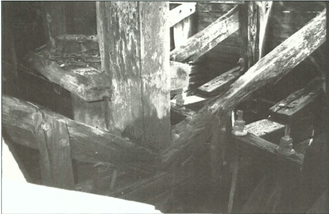
Figure 5-160. Longitudinal stringers spanning one pair of wing frames provide platform to support the vertical discharge pipe. Extra vertical timbers distribute weight of pipe to other horizontal timbers in the wing truss system. Longer longitudinal stringers like that shown in Figure 5-156 provide lateral support to vertical timbers. Port wing, view to the north (forward).
