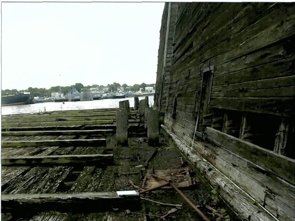
Figure 5-81. View aft (south), showing bilge block stringers in relation to wing and bitt.
