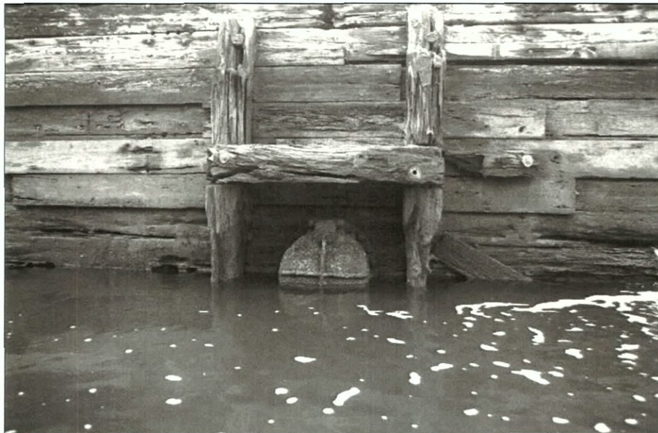
Figure 5-150. Pump outlet on outer hull.
