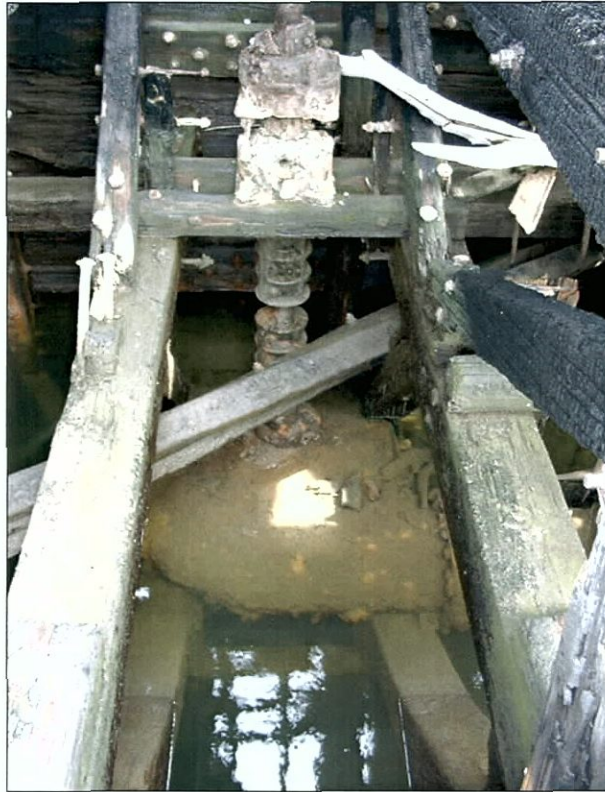
Figure 5-149. One of two impeller casings with vertical drive shaft connected to electric motor on top deck of wing. Port wing, view to the west (port).
