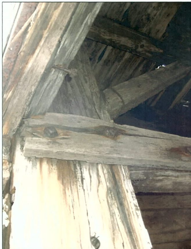
Figure 5-110. Port wing, inner wall truss joint. Note composite horizontal beam. View to the southwest (aft).
