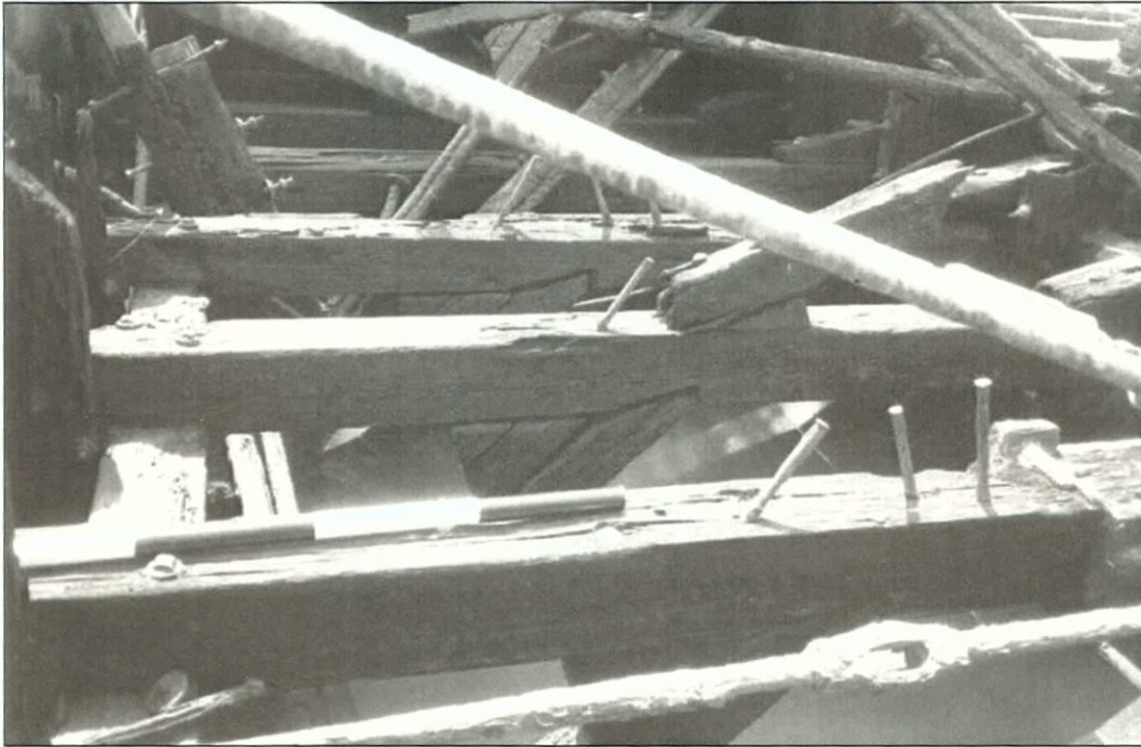
Figure 5-63. Exposed northern end of V1, showing Truss 8 and main deck beam. Note truss attachment under deck beam at center of photo. Also note use of triangular chock. View to the south (aft).
