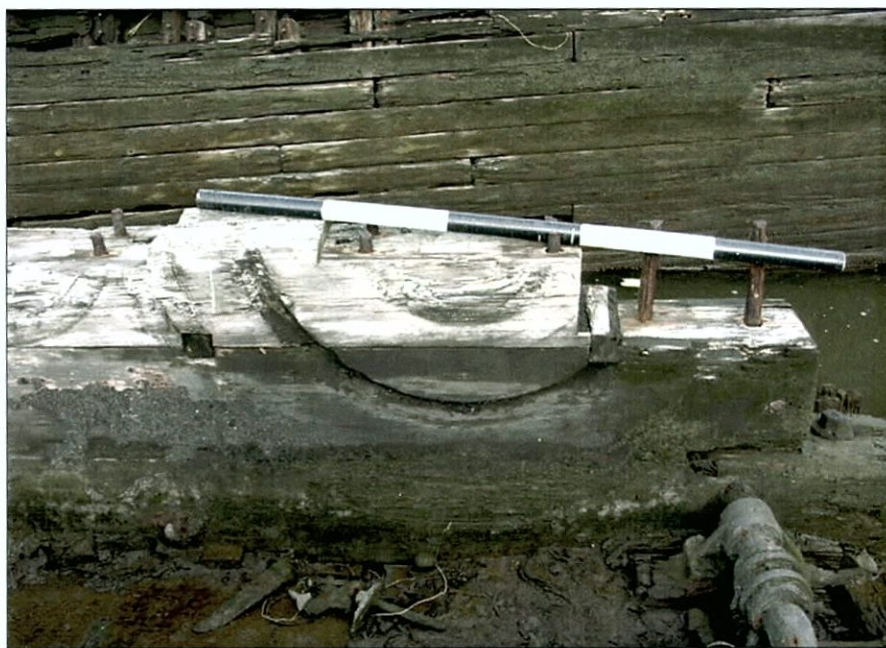
Figure 4-54. Close-up of port side cable mount, showing circular wear from cable spool. View to the east (port).
