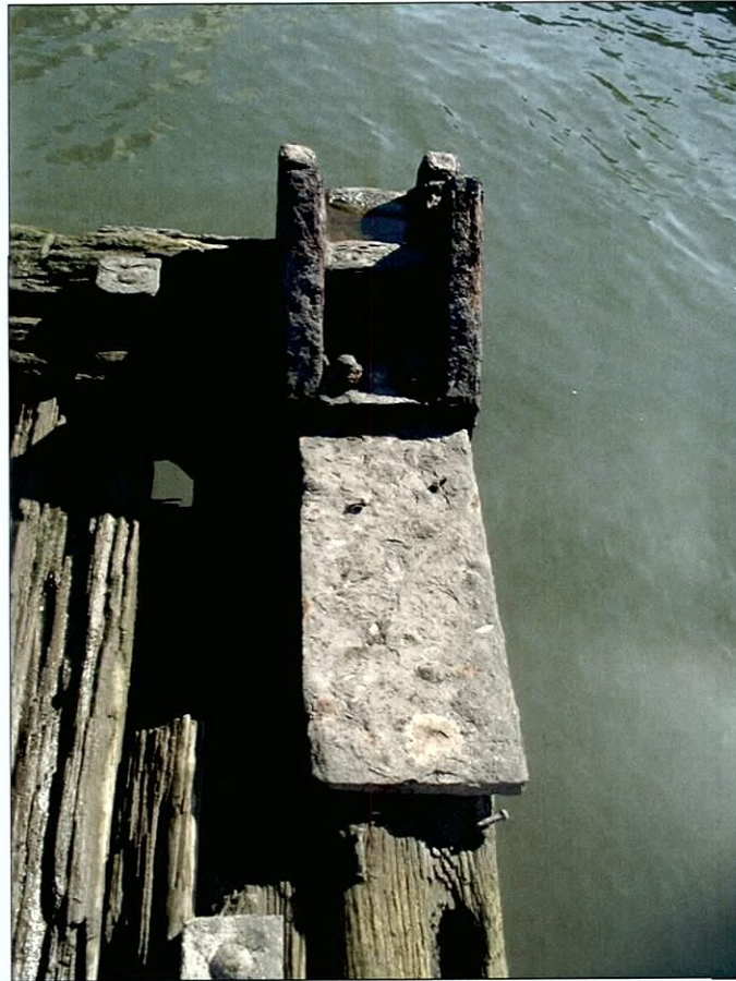
Figure 4-46. Port A-frame mount on starboard hull extension. View to the south (forward).
