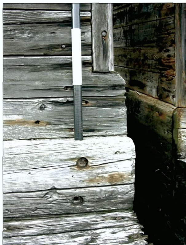
Figure 5-130. Close-up of forward inner corner of port wing, V1. View to the west (port).
