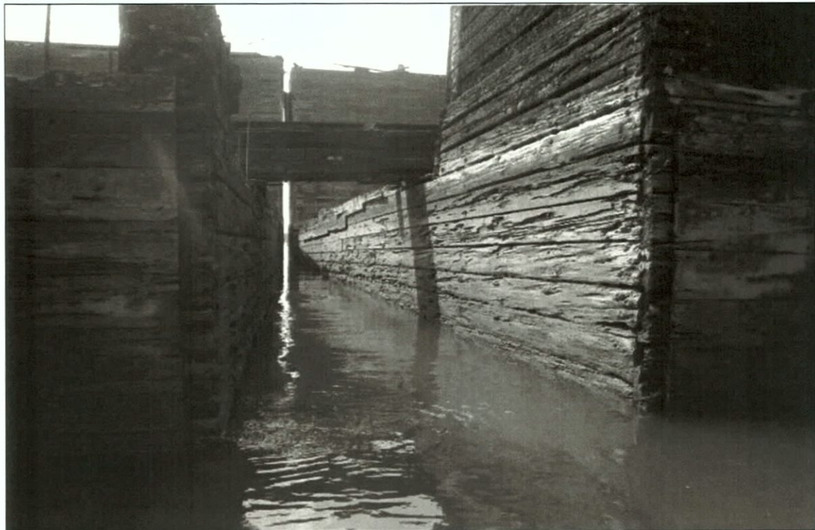
Figure 5-21. Aft edge, with V1 on the left and V2 on the right. View to the west.
