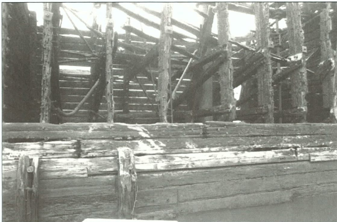
Figure 5-45. View starboard wing showing placement of watertight bulkheads, noted at opposite ends of photograph. View to the west.
