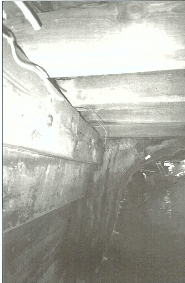
Figure 7-64. Detail of deck beams resting on the clam and shelf along with a hanging knee. Looking aft (north).
