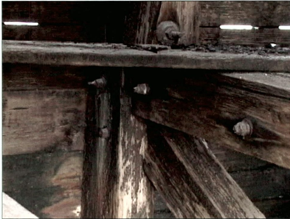
Figure 5-98. Outer wall wing framing at upper deck, port wing. Note deck planking.
