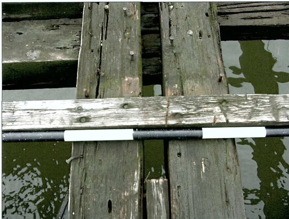
Figure 6-83. Single remaining deck plank just starboard of forward hatch. Note rose head spikes and fastener pattern.
