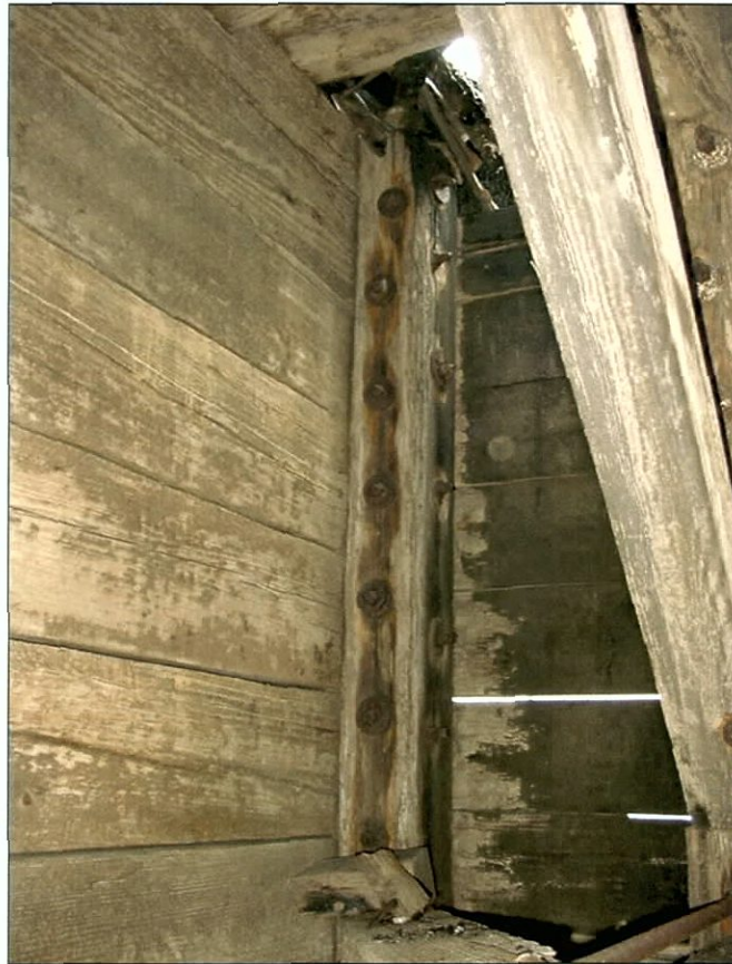
Figure 5-48. Intersection of bulkhead and outer hull in port wing. View to the northwest (port forward).
