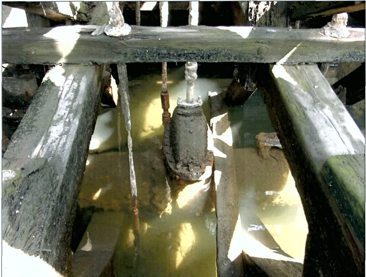
Figure 5-151. Gate valves in inlet (below) and outlet (center) pipes. Port side, view to the west.
