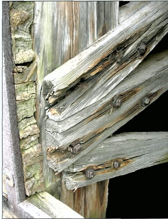
Figure 5-107. Inner wing wall frame with truss timbers fastened. Note lower timber is notched rather than composite. View of starboard wing, view to the south (aft).
