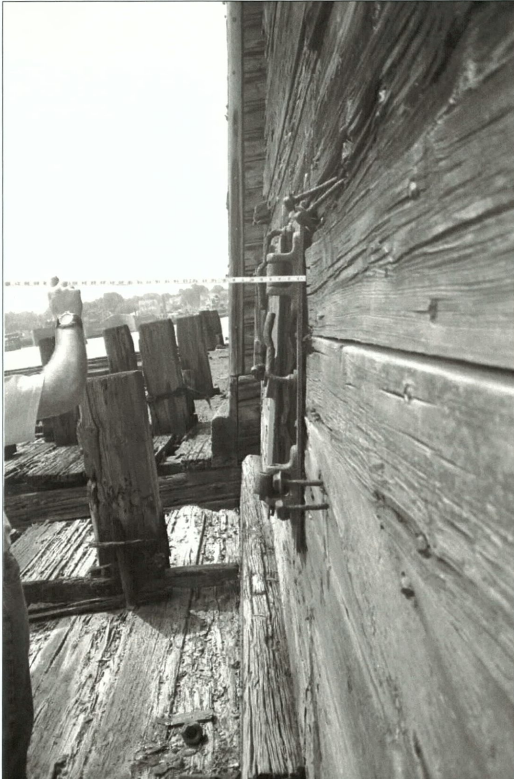
Figure 5-142. Aft small hatch, port wing side detail. View to the south (aft).
