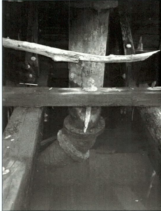
Figure 5-158. Base of vertical discharge pipe. Port wing, view to the west (port).
