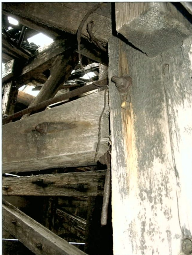
Figure 5-111. Opposite side of joint in Figure 5-110. Note iron fastener. View to the northwest (forward).
