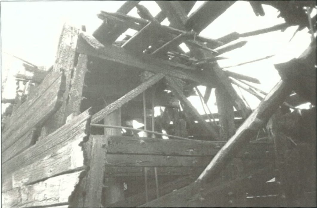
Figure 5-102. Wing truss at upper deck level. Starboard wing. View to the northeast.
