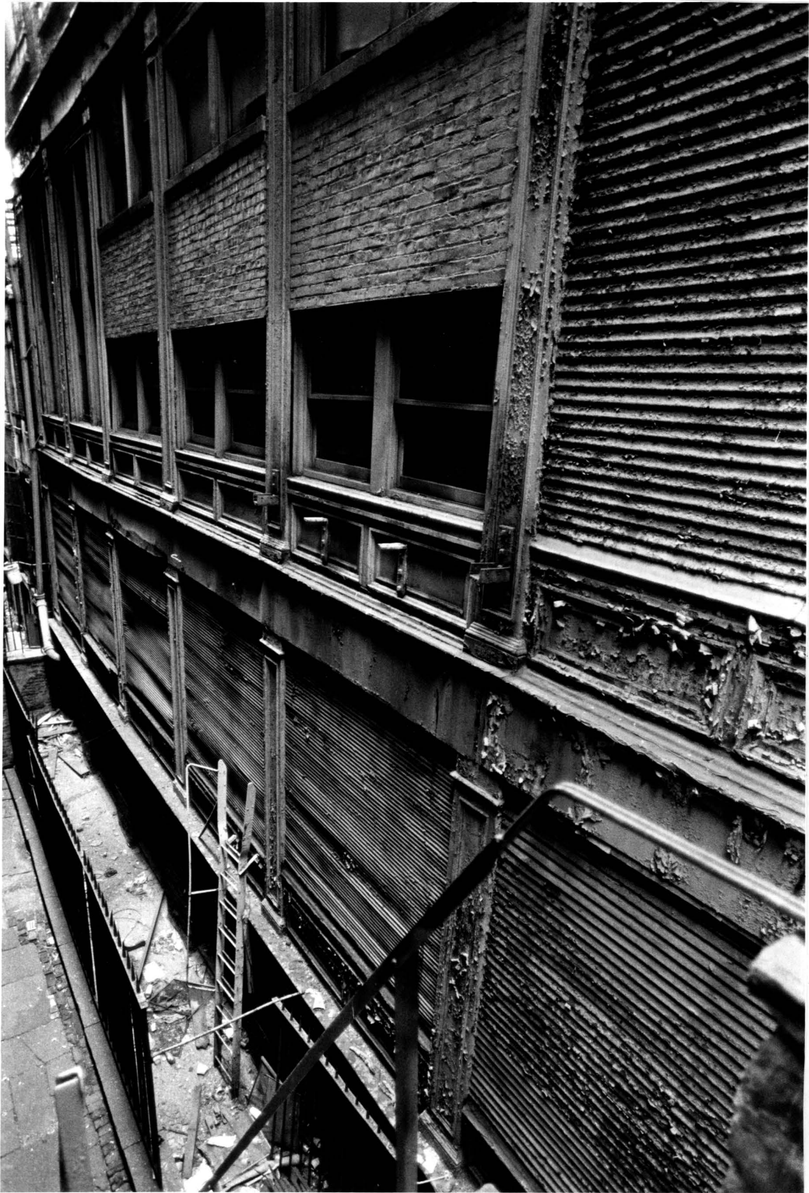
55 White Street View of basement and first-story rear elevations Photo: Carl Forster
