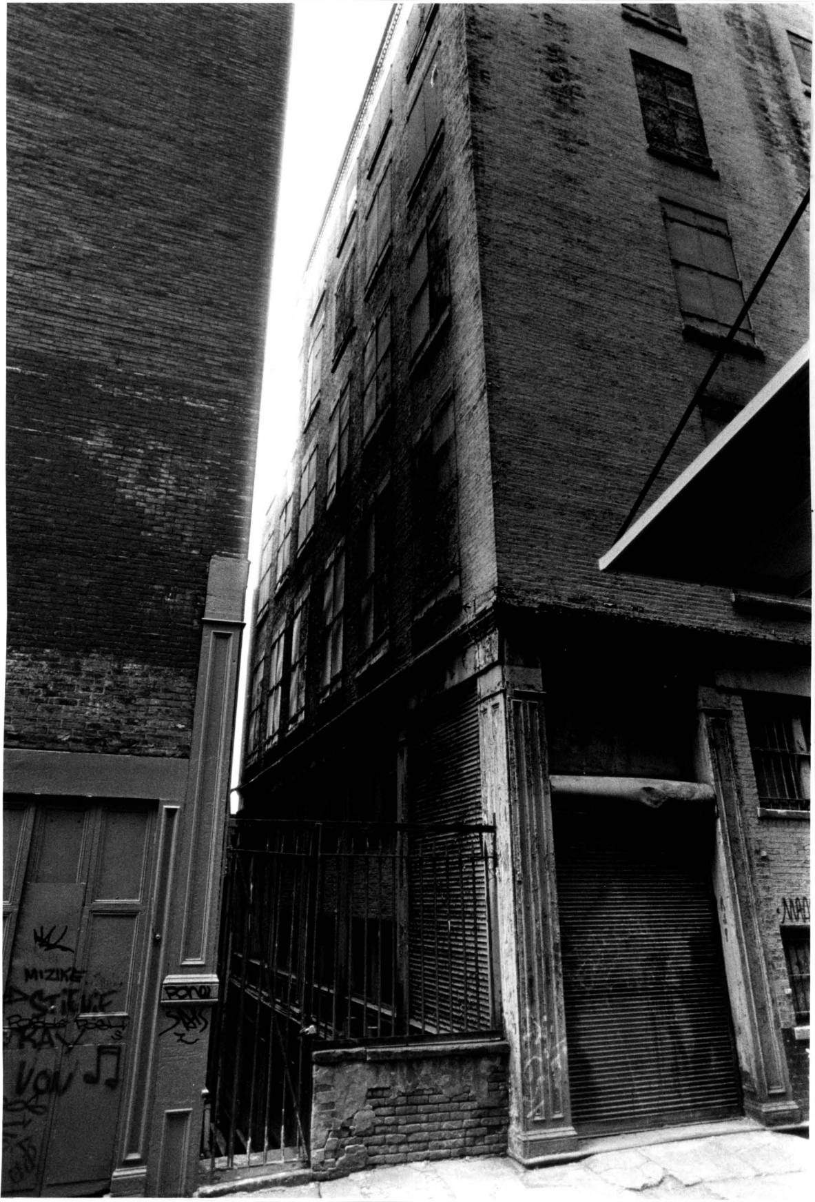
55 White Street View of the Franklin Place and rear elevations Photo: Carl Forster
