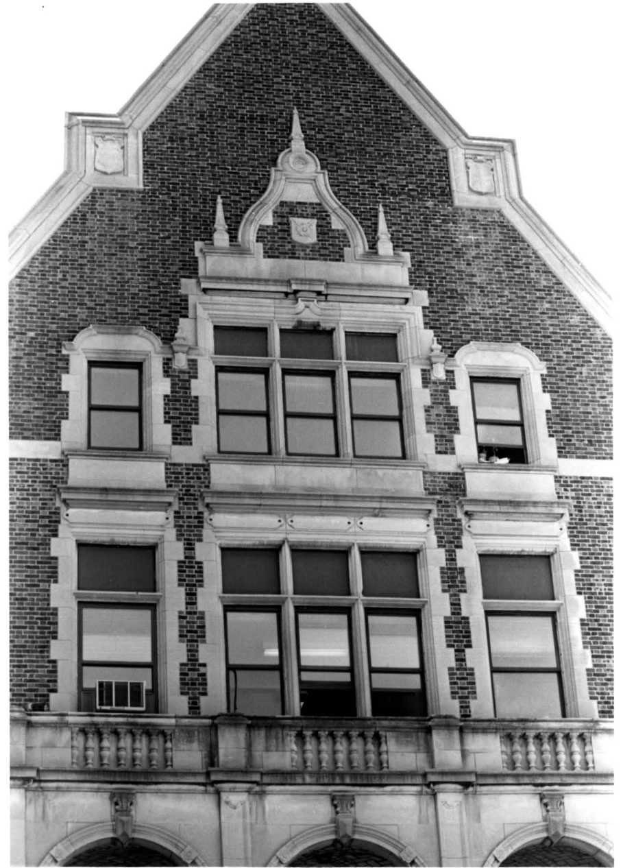
Messiah Home for Children Detail above porch, West Tremont Avenue elevation Photo: Carl Forster
