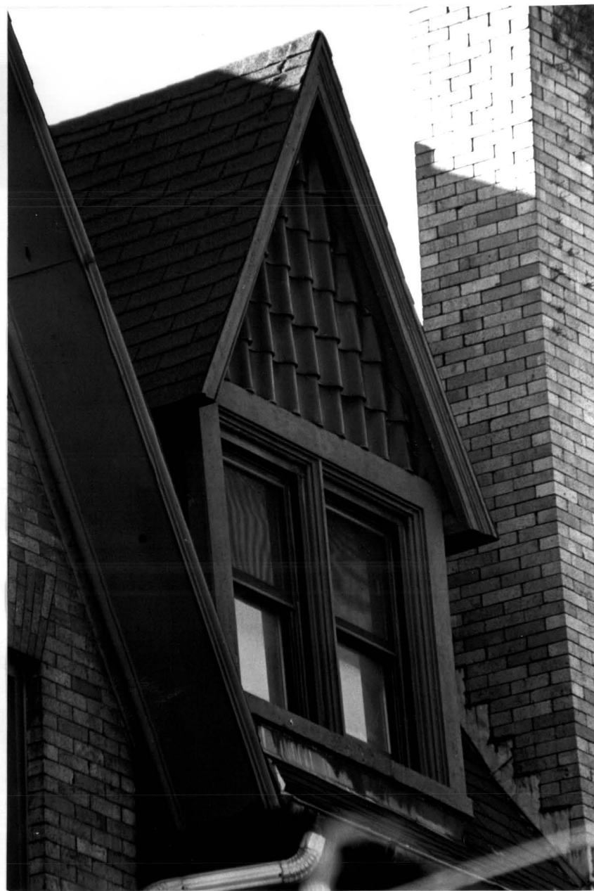
Nicholas C. and Agnes Benziger House North facade, west dormer Photo: Carl Forster
