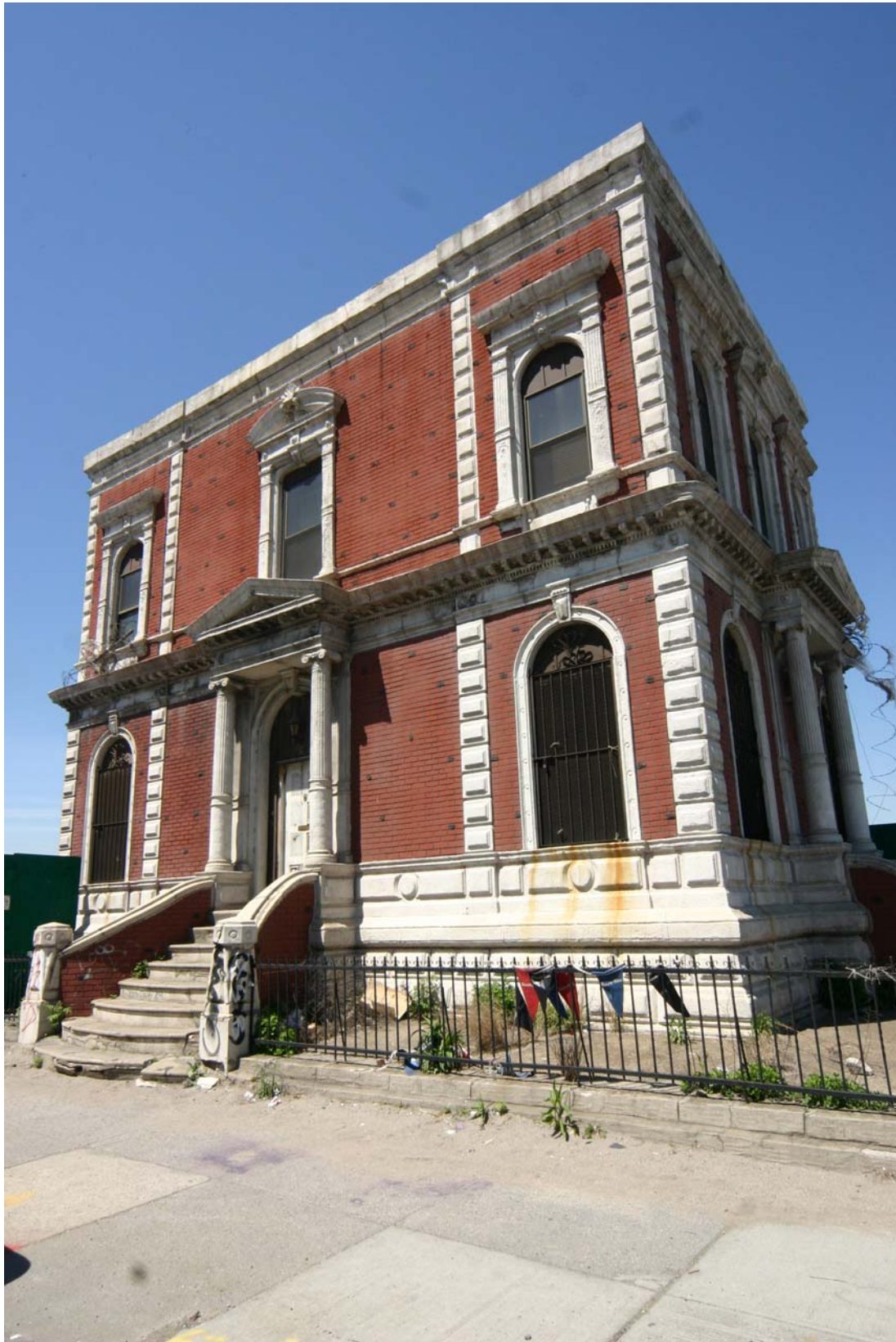
New York and Long Island Coignet Stone Company Building Third Avenue facade Photos: Carl Forster
