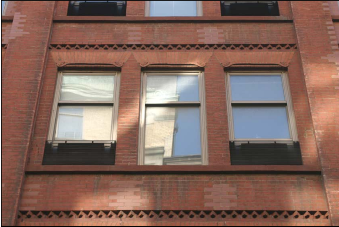
F.W. Devoe & Co. Factory Detail of typical bay Photo: Christopher D. Brazee (2008)
