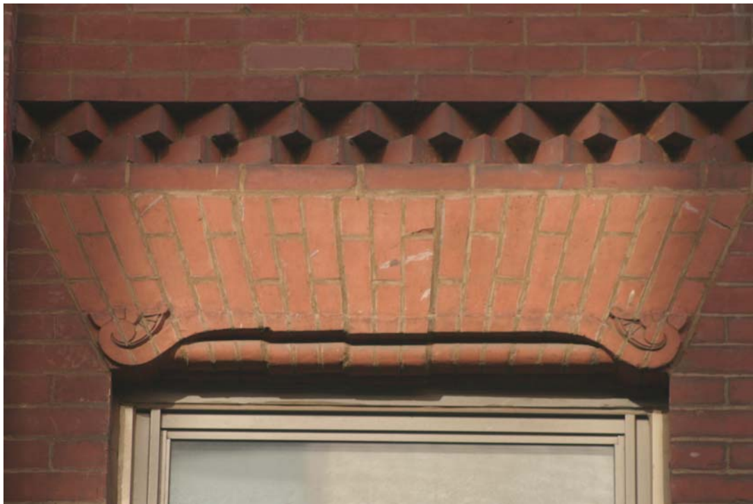
F.W. Devoe & Co. Factory Detail of terra-cotta window lintel and sawtooth brickwork Photo: Christopher D. Brazee (2008)
