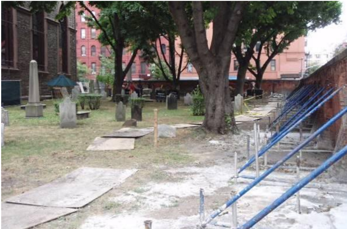
Photograph 1 – Inside of Old St. Patrick’s Cathedral Brick Wall. Photograph parallel to Prince Street facing east toward Mott Street.
