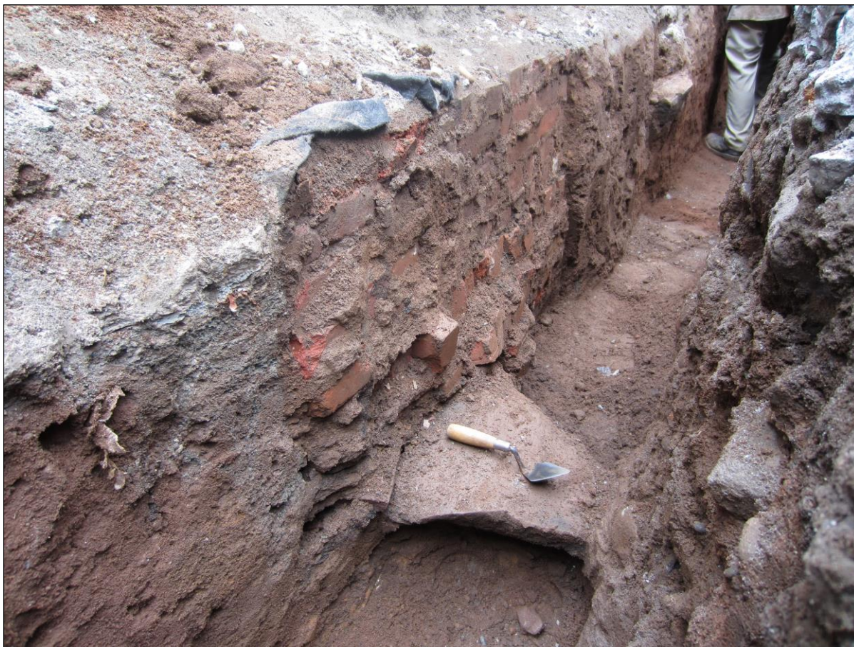
Image 08: Excavation the northern edge of Feature 4 as part of the water line excavation trench.
