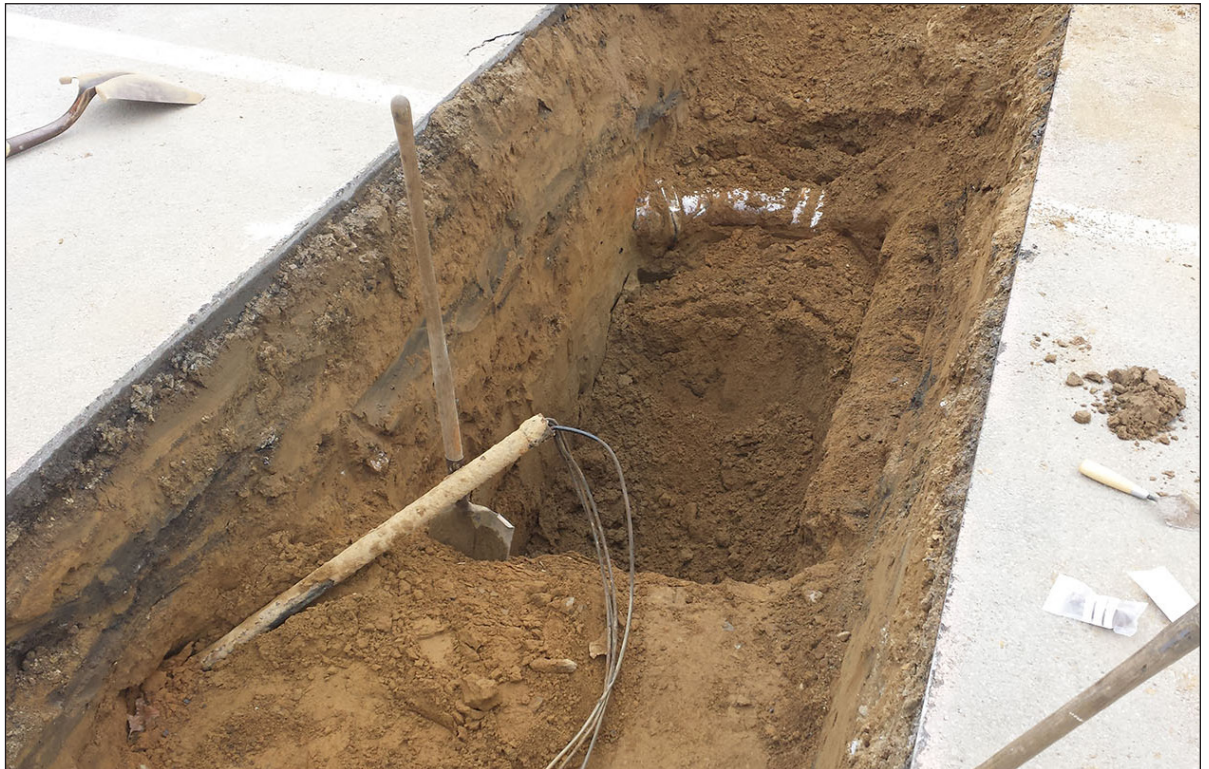
Facing southeast showing completed Trench 1. Note electrical conduit extending from wall towards bottom of photo and water line in background 4
