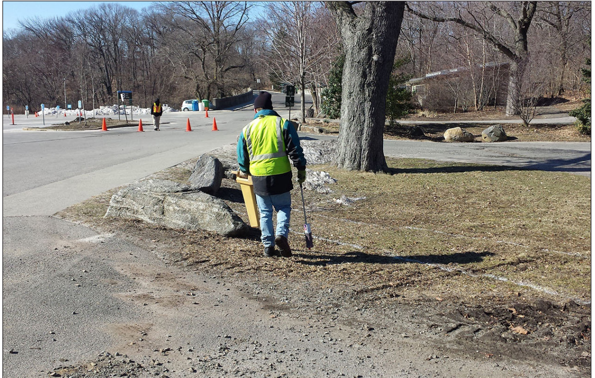
Facing south from north edge of Lot B showing utility mark out for Trench 6. Lot B parking lot is to the left 1
