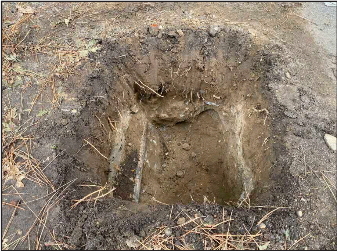
Photograph B.5. View facing northwest showing the excavation for Sign 12. Note the electrical conduit running along the southwestern edge of the excavation (Photographer: James Lee, October 2019 [HRI Neg.#19070/D1:032]).
