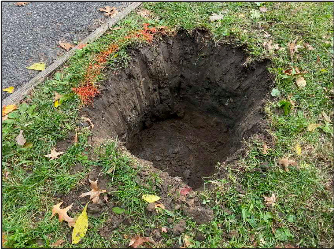
Photograph B.4. View facing northeast showing the excavation for Sign 8. Bedrock was encountered at the base of the excavation (Photographer: James Lee, October 2019 [HRI Neg.#19070/D1:077]).
