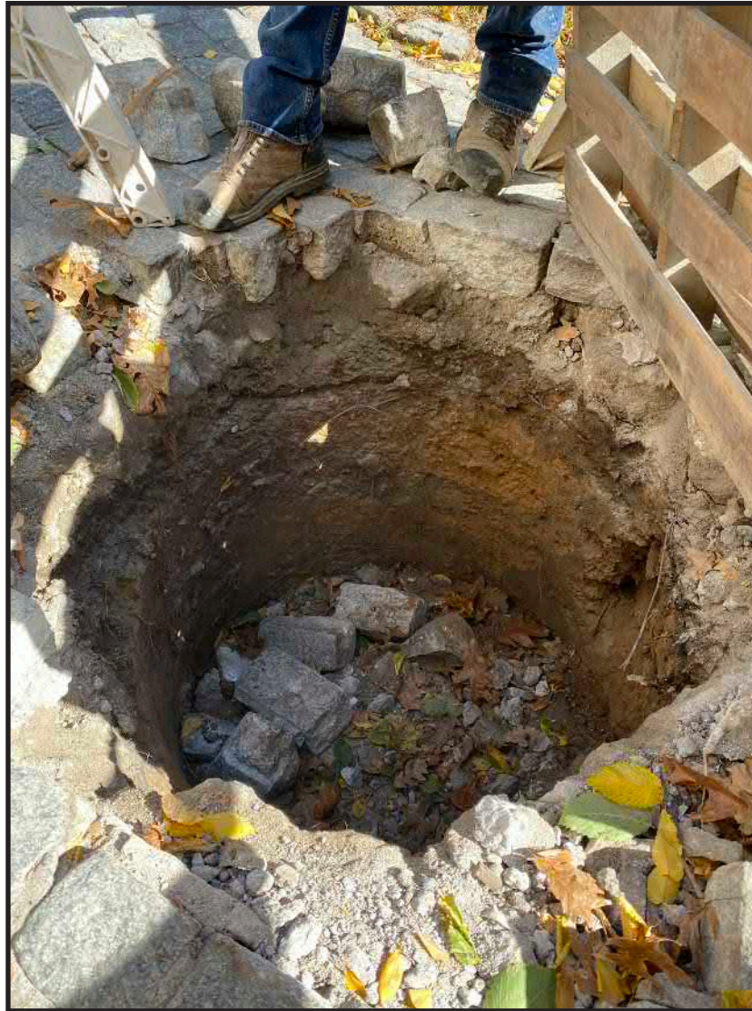
Photograph B.2. View facing northeast showing the excavation for the kiosk (Photographer: James Lee, October 2019 [HRI Neg.#19070/D1:084]).
