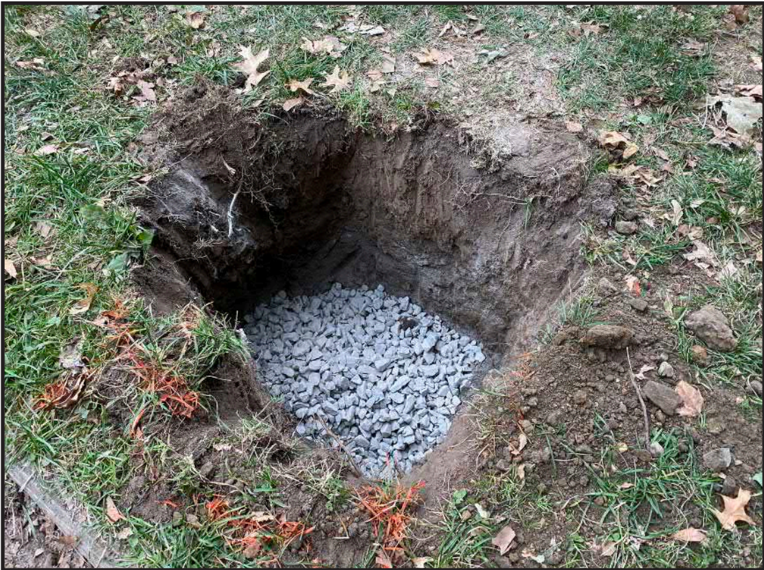
Photograph B.1. View facing northeast showing the completed excavation for Sign 13 (Photographer: James Lee, October 2019 [HRI Neg.#19070/D1:022]).
