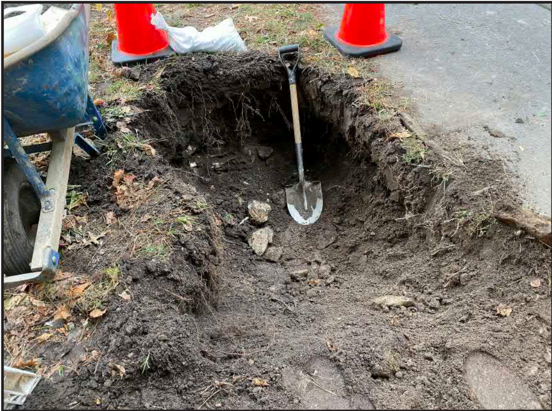
Photograph B.8. View facing north showing the large excavation necessary for the eastern introductory sign. Note the rocky context present below the topsoil (Photographer: James Lee, October 2019 [HRI Neg.#19070/D1:039]).
