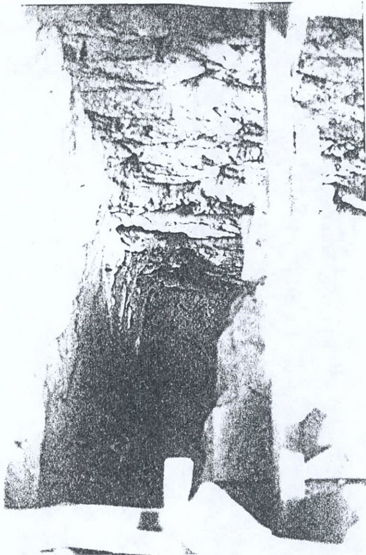
Plate 26 Intersection of Northeast Foundation Wall of Main Wing and East Foundation Wall of Hyphen View South Looking Downward From Hyphen Porch
