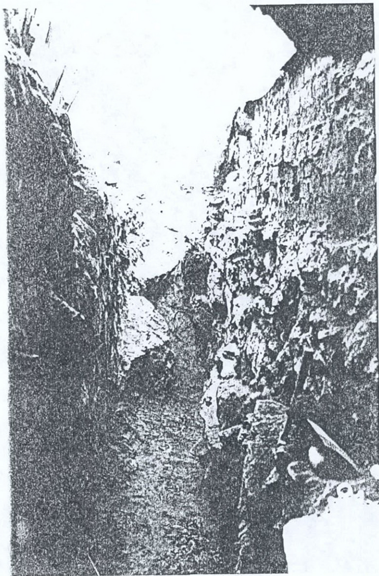
Plate 13 North Foundation Wall of Mansion Exposed East of Hyphen Note Blue Material on Wall Applied During Waterproofing View East
