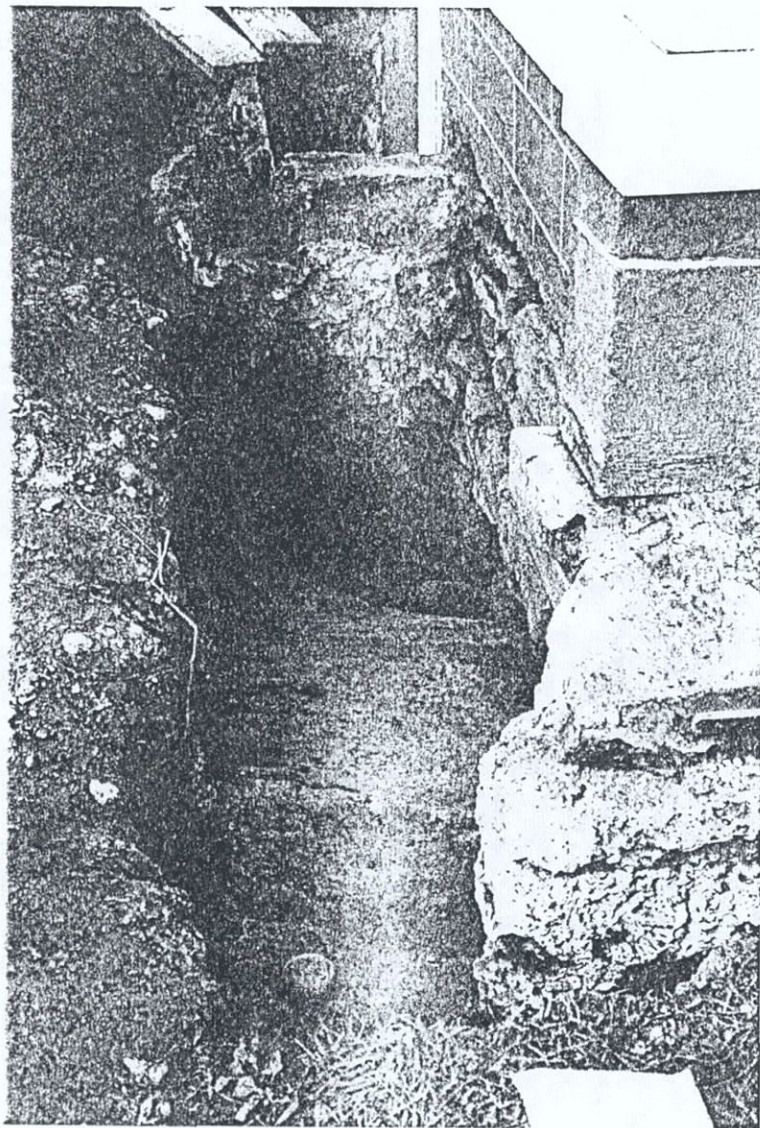
Plate 21 Northwest Corner of Mansion Foundation Wall Resting on Bedrock Slab View East
