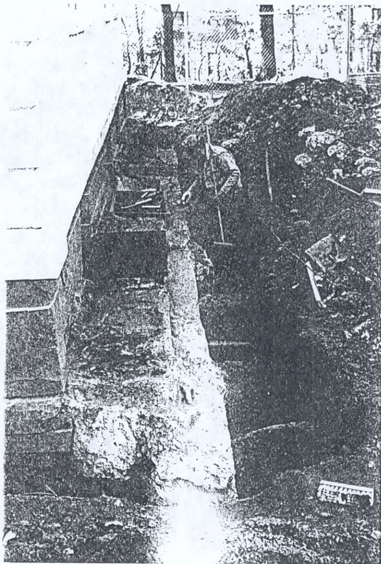
Plate 16 West Side of Mansion Showing Area Next To Foundation Disturbed by Areaways, Concrete Slabs and Pipe Trenches View South
