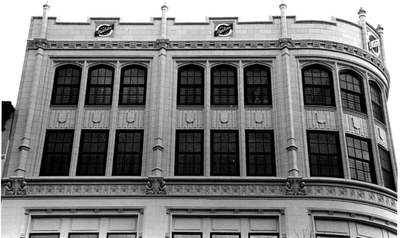
Studebaker Building, Bedford Avenue facade, fourth and fifth stories Photo: Carl Forster
