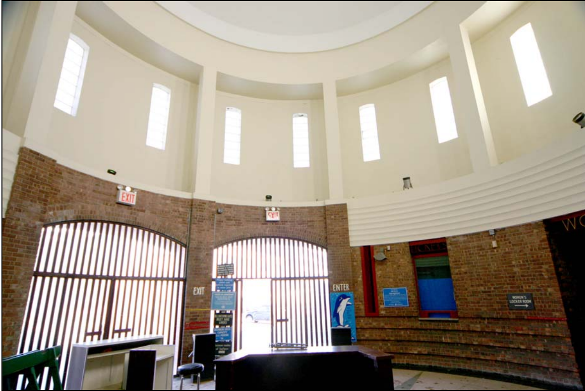
Tompkinsville (Joseph H. Lyons) Pool Bath House Interior: Entrance and Ticket Booth Photo: Carl Forster, 2007
