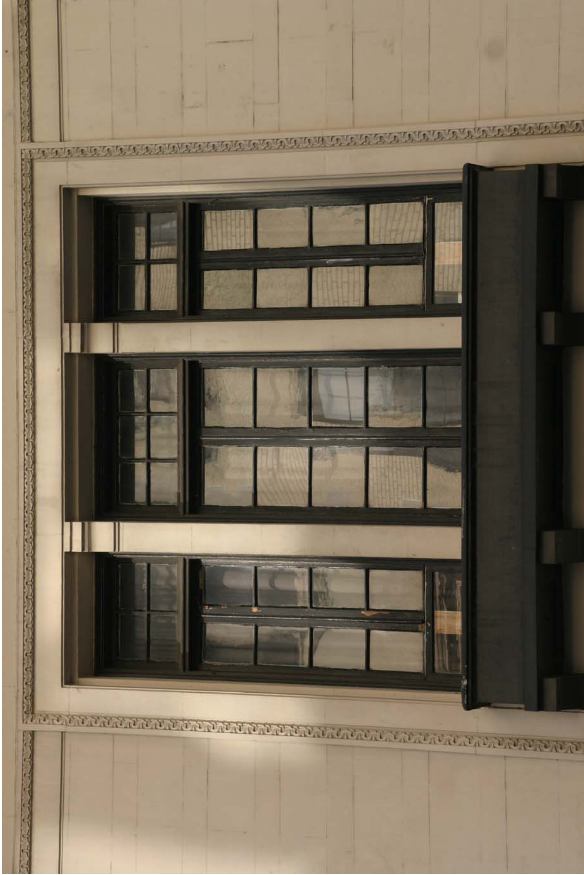
E. Hayward and Amelia Parsons Ferry House Third-story windows Photo: Christopher D. Brazeel, 2008
