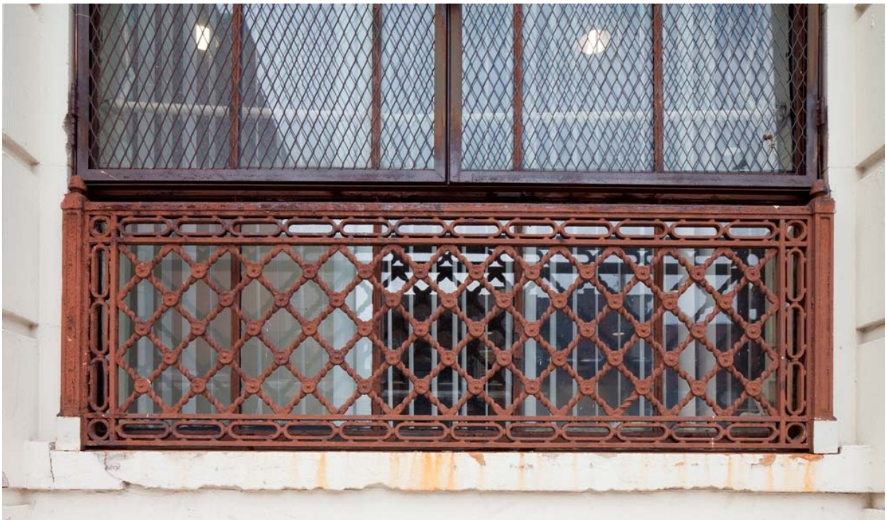
Williamsburg Branch, Public National Bank of New York (now Bank of America), Graham Avenue façade panel detail Varet Street façade metal grille detail
